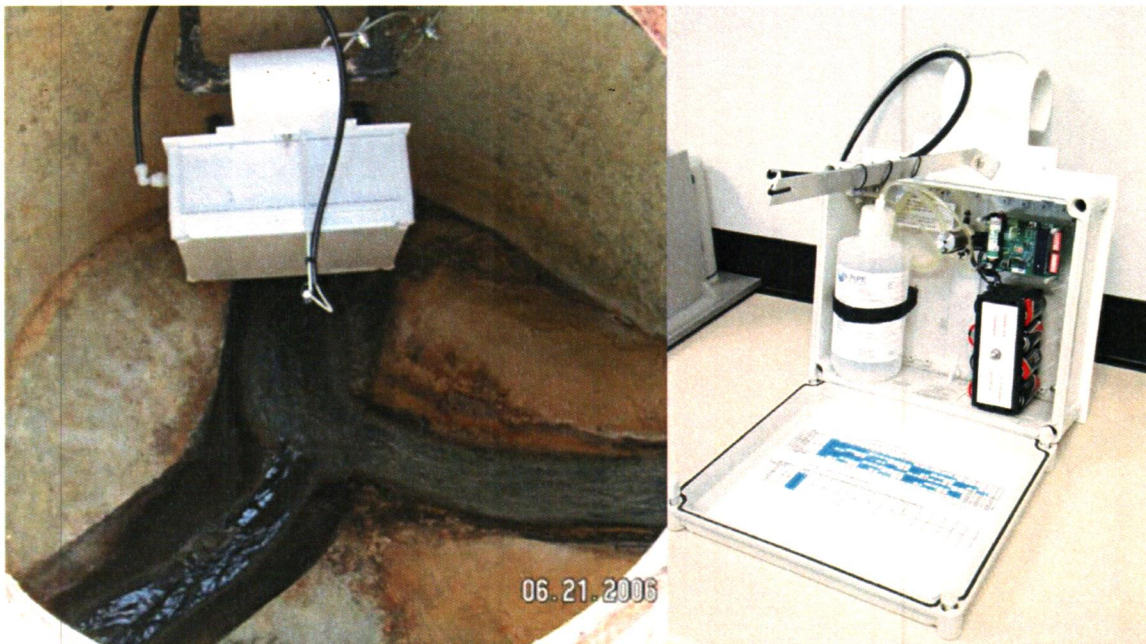
Figure 2 Bioaugmentation Program in the Collection System (left) and In-Pipe G 2 MDU
