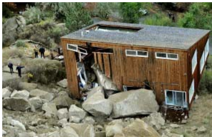
Figure 9. Private and Public Structures Affected by Landslides
