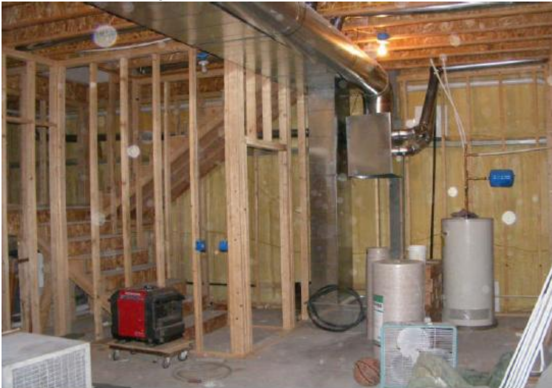
Garage Interior – Lower Level – Mechanical Area
