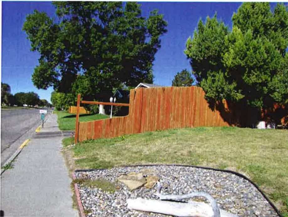
Looking west from subject property at fence between subject property at 2107 Colton Blvd. and neighboring property at 2111 Colton Blvd. Fence has structure above 30" in the Clear Vision Area and a portion of the fence is above the 4' in front yard setback of 20'
