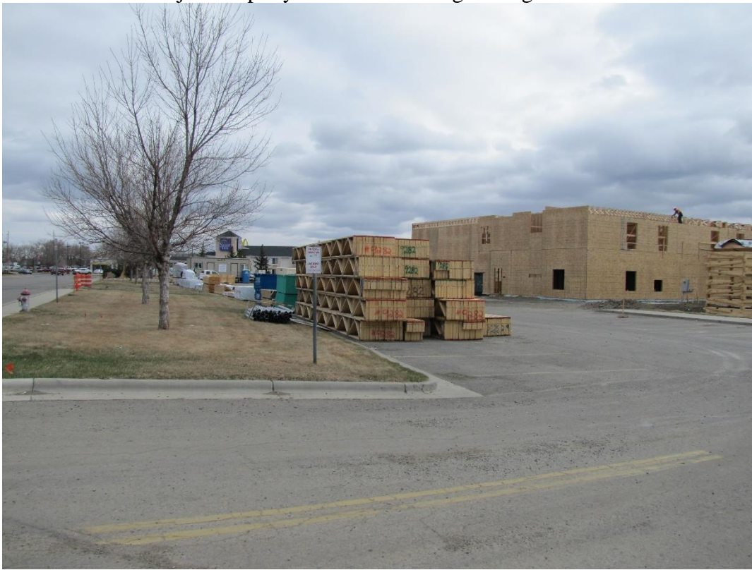
View east along Southgate Dr – Comfort Inn and Suites under construction at 4908 Southgate Dr
