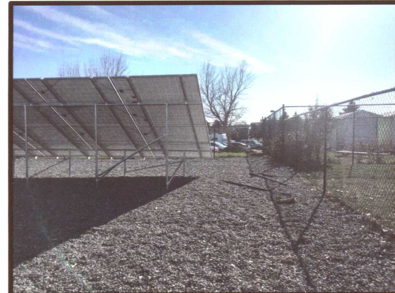
PHOTO 5: SOUTHERN PHOTOVOLTAIC ARRAY, STANDING AT WESTERN PERIMETER OF FENCED AREA, LOOKING SOUTH.
