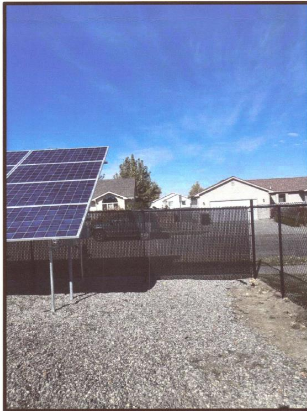
PHOTO 4: NORTHERN PHOTOVOLTAIC ARRAY, STANDING AT EASTERN PERIMETER OF FENCED AREA, LOOKING NORTH.
