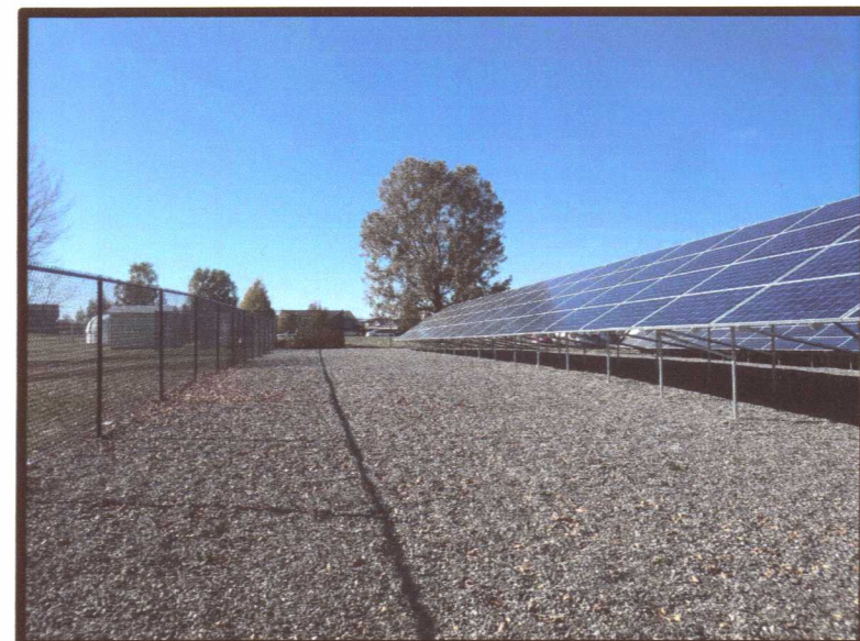
PHOTO 6: SOUTHERN PHOTOVOLTAIC ARRAY, STANDING AT EASTERN PERIMETER OF FENCED AREA, LOOKING WEST.
