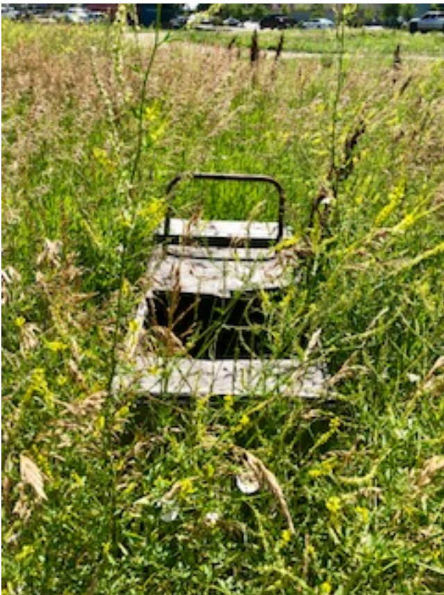
View of debris on North end of A35427
