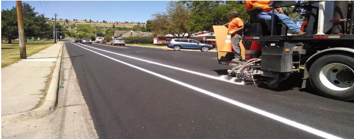
Image 2.3 Installation of bike lane as part of restriping project of 13 th Street West in July 2014
