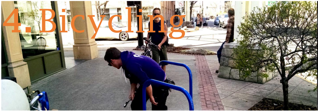
A member of the public waits for Downtown Business Improvement District staff finish the installation of two city bike staples so he can park his bicycle.
