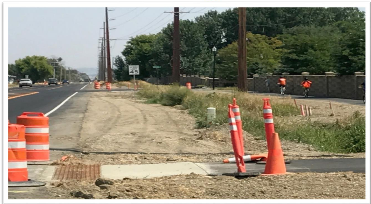
Complete Street Elements being constructed as part of the Grand Avenue and 56 th Street West reconstruction project as part of the new Ben Steele Elementary School
