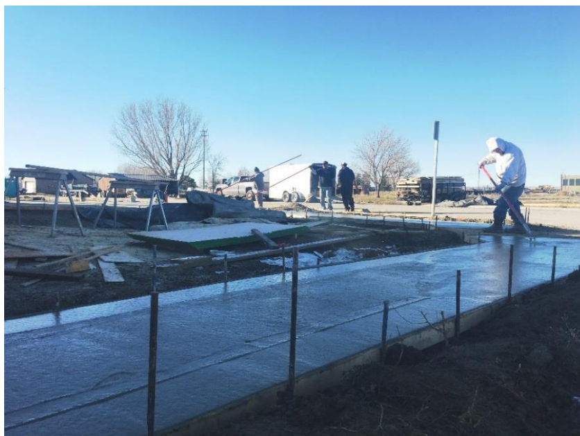
Image 1.1 Construction crews building boulevard sidewalks as a requirement for a new subdivision hence preventing increased installation costs in the future
