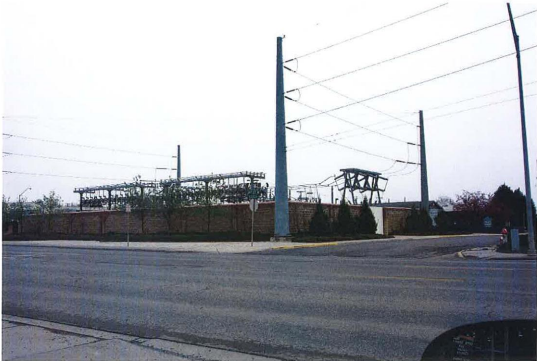
Northwestern Energy Substation on 24 th Street West looking northeast.
