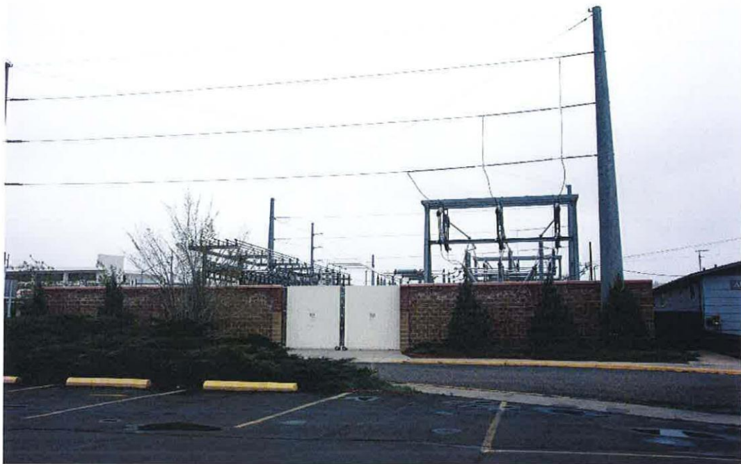
Existing Northwestern Energy Substation near Grand and 24 th intersection. This view is from the south side of the station looking north from Alderson Avenue.
