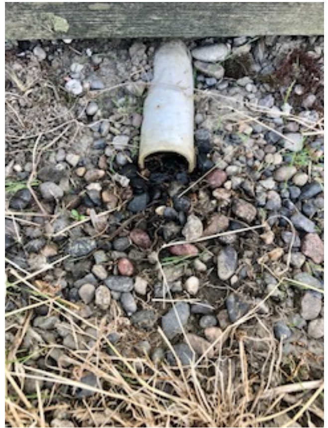
View of shop floor drain 2 discharge – north side of shop
