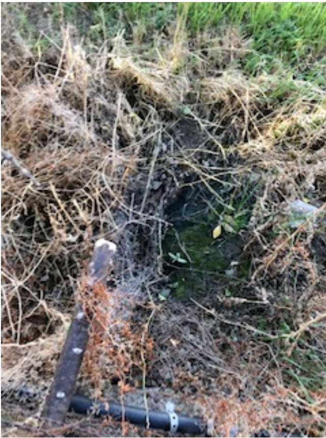
View 3 of GW well line – north side of home – terminus
