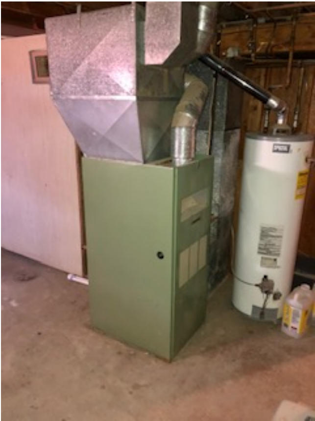
View of gas home and water heaters – floor drain -
