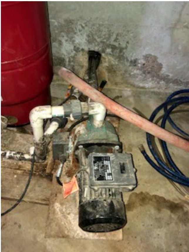
Close-up view GW well pump with suction line exiting home
