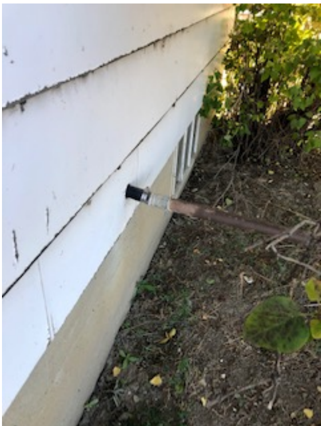
View of out of use GW well line – north side of site home
