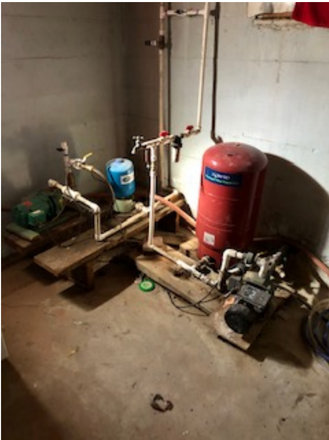
View of groundwater well pumps in NE corner of basement
