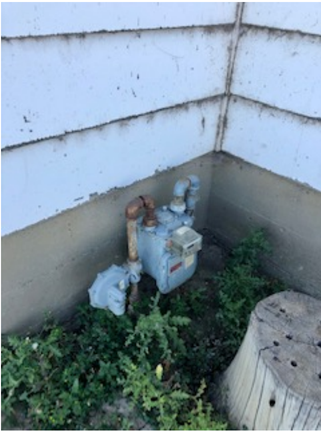
View natural gas meter – east side of site home
