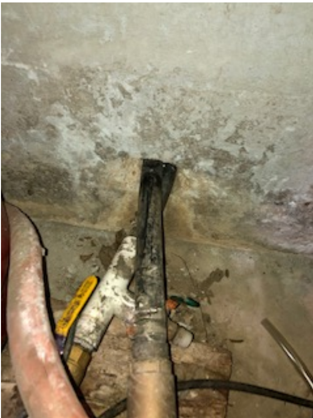
Close-up view 2 of suction line for GW well pump
