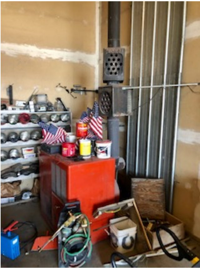
View of gas heater – NE corner of shop interior
