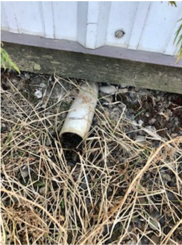
View of shop floor drain 1 discharge – north side of shop
