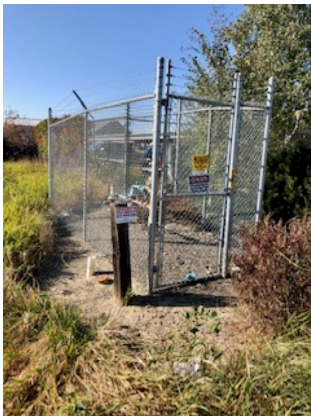
View of gas pipeline valve station – adjacent to site and north
