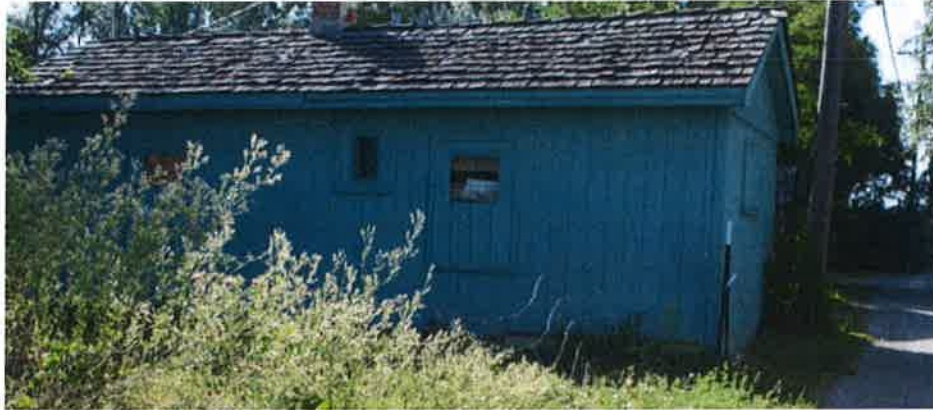
Subject: 910 South 27 th Street, Billings, MT 59101 Description: North and west sides of the detached shed along the alley
