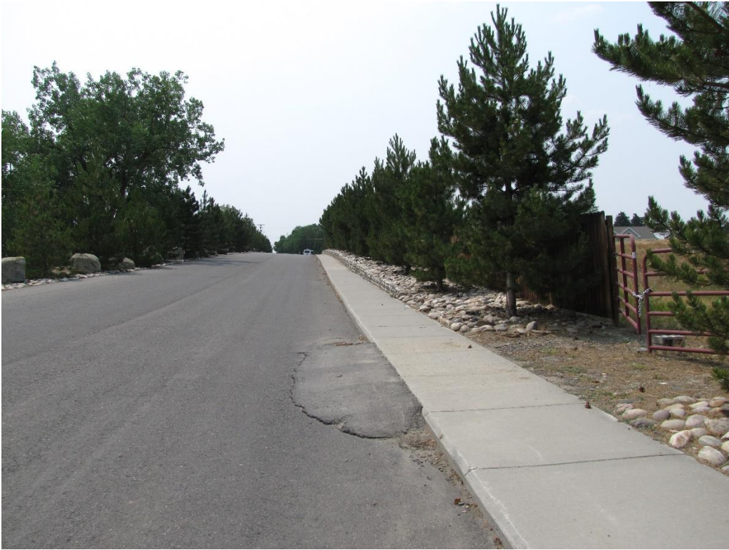
View west along southern leg of Cherry Creek Loop – subject property on the right
