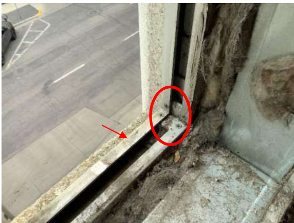
Photo #35 Exterior window frame piece indicated by red arrow attached to main frame by plate at the corner indicated by red oval.
