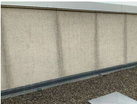
Photo #17 Discoloration of the penthouse precast wall panels adjacent to the sealant joints.
