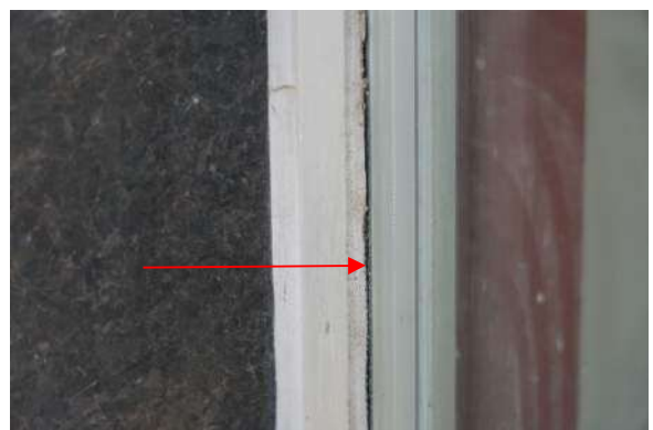
Photo #42 Failed glazing sealant at the first floor fixed windows indicated by red arrow.
