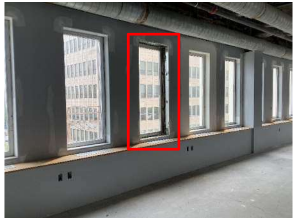
Photo #10 Gypsum board had not been installed at one window on the fourth and fifth floors indicated by the red rectangle.
