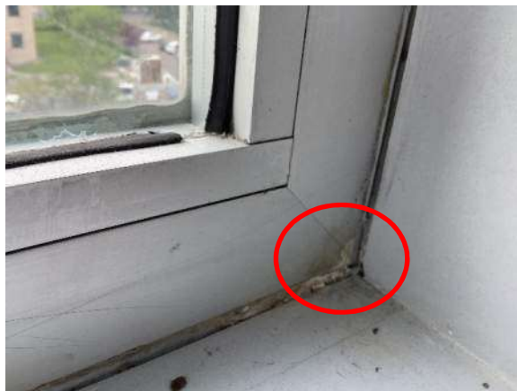
Photo #39 Staining consistent with water leakage originating at the corner of the sash indicated by red oval
