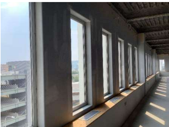
Photo #25 Typical interior view of the operable window units installed at floors two thru five.
