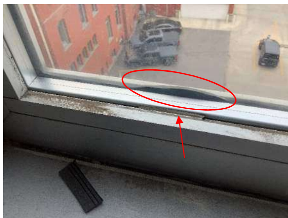
Photo #53 Butyl glazing tape bulging from the exterior glazing joint (red oval) at the shim (red arrow).
