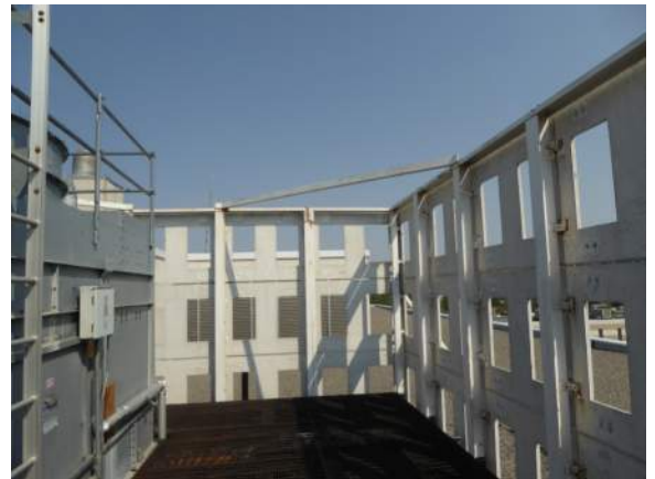
P42: Roof top mech equipment enclosure; precast concrete panels and steel frame
