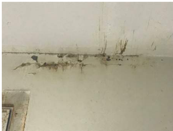
P22: Concrete cracking with delamination near top of wall at north side of the parking garage
