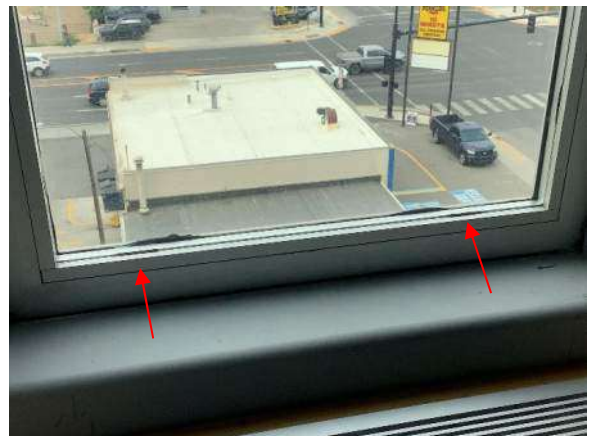
Photo #52 Butyl glazing tape bulging from the exterior glazing joint at the shim locations indicated by the red arrows.
