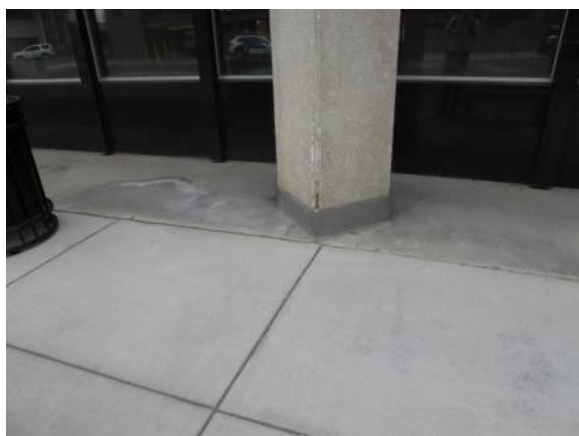
P5: weathered façade
