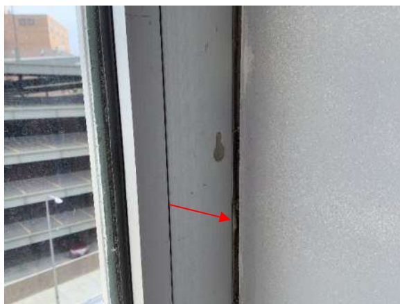
Photo #27 Sash latch key holes have been filled with sealant. Sash crack is visible behind drywall indicated by red arrow.
