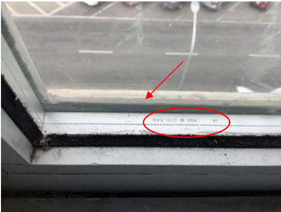
Photo #31 Exterior glazing sealant at circa 1991 IG unit replacement (red arrow). Note "91" IGCC spacer stamp (red oval).
