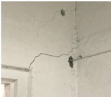
P29: concrete wall crack
