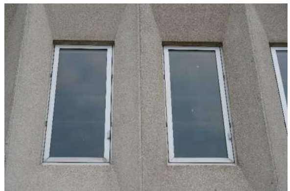
Photo #24 Typical exterior view of the operable window units installed at floors two thru five.
