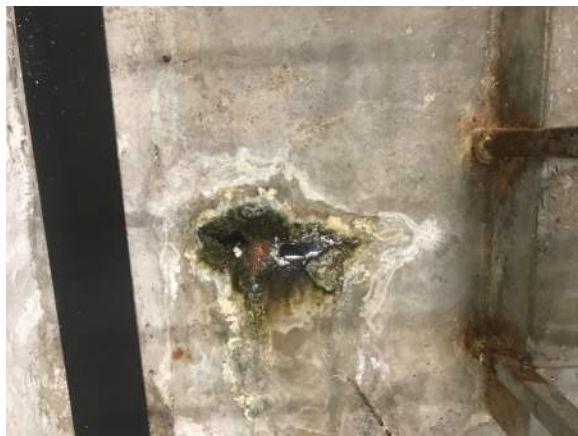
P24: floor spall and leaking fluids
