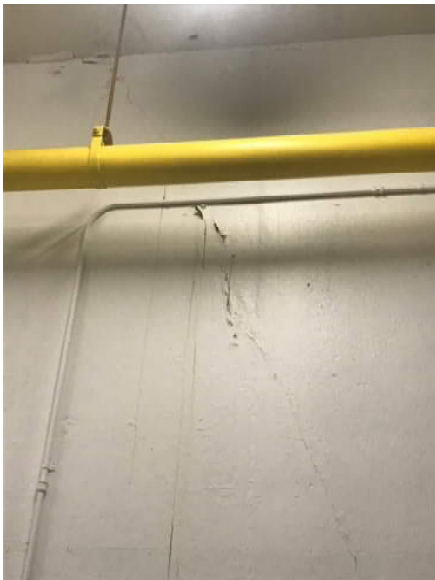
P27: concrete wall crack
