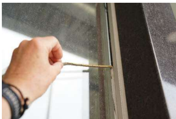
Photo #41 Original compound glazing overcaulked with polyurethane sealant at the first floor.
