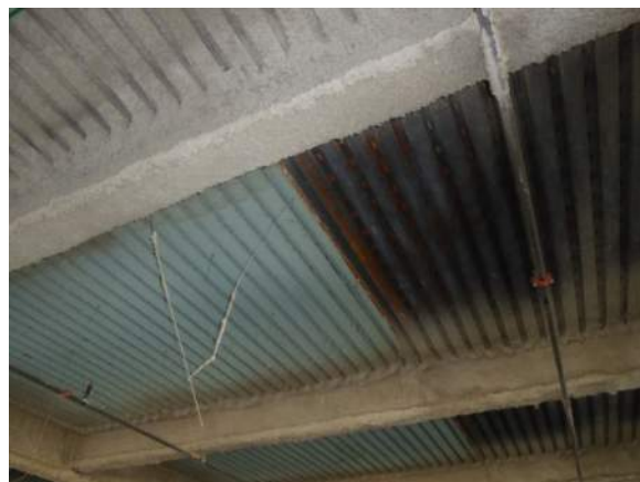
P34: blue fire protection with deck corrosion
