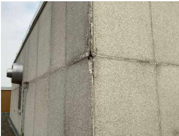
Photo #15 Area of concrete deterioration at the southwest corner of the penthouse.
