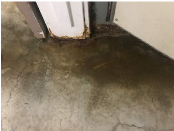
P30: floor stain; possibly moisture intrusion
