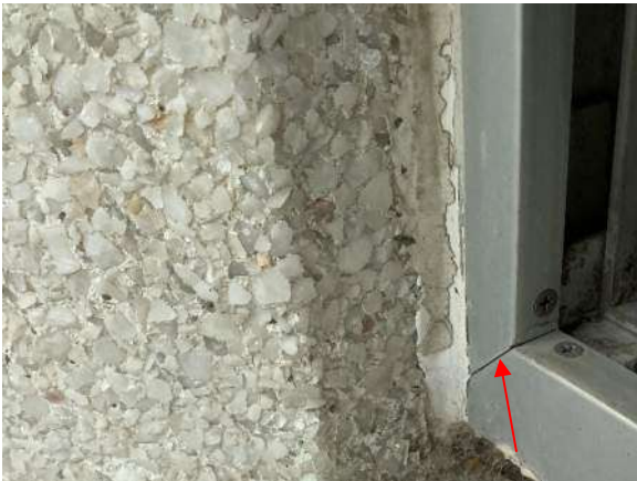
Photo #55 Overcaulked window perimeter sealant at the fourth floor. Note that the frame corner joint is open (red arrow).
