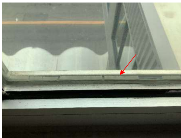
Photo #29 Original compound glazing was observed to be in very poor condition from the building interior indicated by red arrow.
