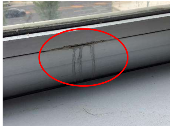
Photo #38 Staining consistent with water leakage originating between the glazing stop and the sash indicated by red oval.
