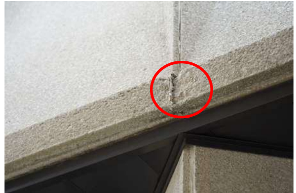
Photo #14 Small area of apparent freeze-thaw damage at the second-floor eyebrow indicated by the red oval.
