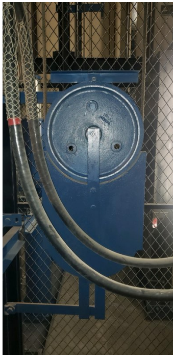
Traveling cables are in good shape with no visible wear.
