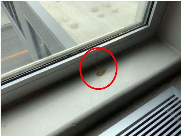
Photo #37 Staining consistent with water leakage originating between the glazing stop and the sash indicated by red oval.
