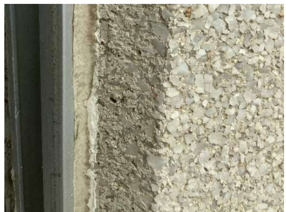
Photo #54 Window perimeter sealant at the fourth floor. Two colors of sealant indicate that the sealant has been overcaulked.
