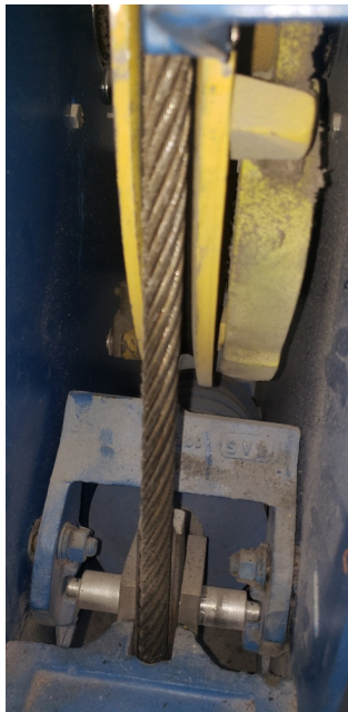
Governor Rope. No presence of rogue (rust) and not worn.
