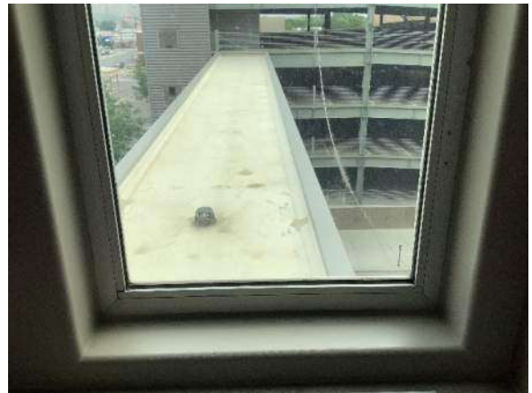
Photo #46 Broken IG unit at the east elevation on the fourth floor.
