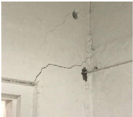
P29: concrete wall crack
