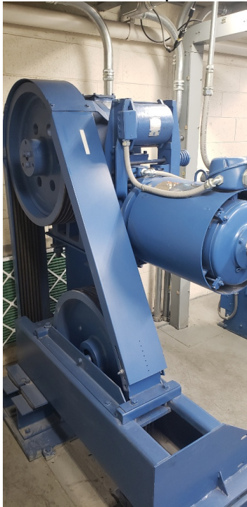
Machine, motor, cables, etc. All in good condition and functionally sound
