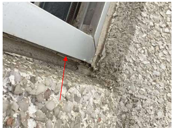
Photo #36 Approximate location of the weep hole is indicated by red arrow.
