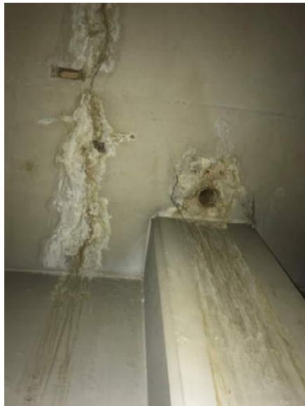
P19: Concrete cracks & stains with efflorescence
