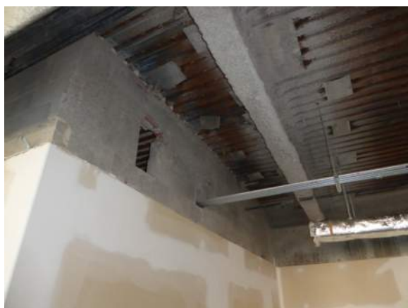
P37: Masonry room with deck corrosion
