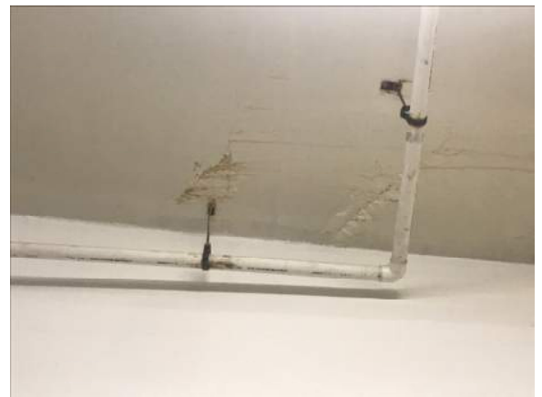
P25: ceiling concrete cracks
