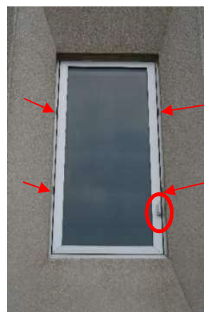
Photo #28 Exterior handle indicated by red oval and latch strike plates indicated by red arrows.
