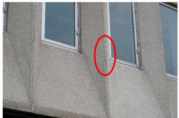
Photo #12 Small crack in precast concrete wall panel indicated by red oval.
