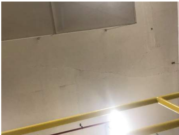
P31: concrete slab ceiling crack
