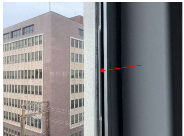
Photo #48 Desiccant-filled tube (red arrow) typical of original IG units.
