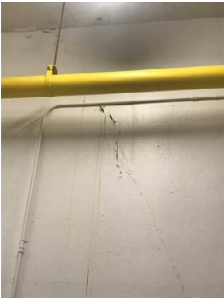
P27: concrete wall crack
