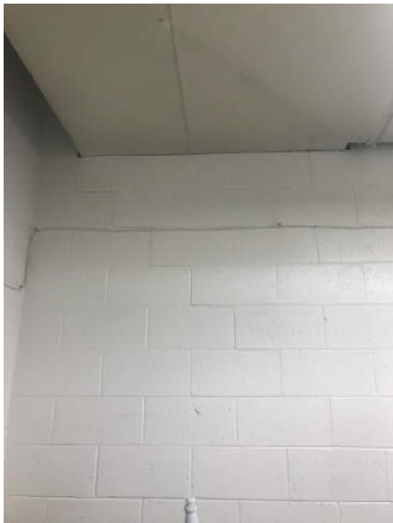
P26: masonry wall crack
