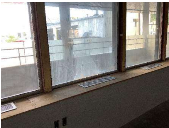
Photo #47 Broken IG unit at the west elevation on the first floor.
