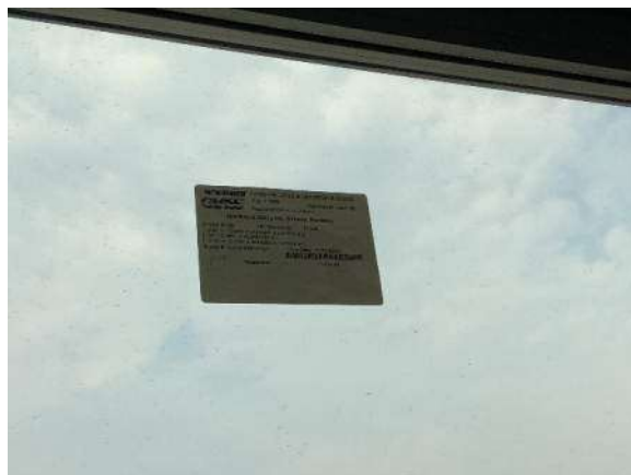
Photo #50 Fabricator sticker found on a number of recently replaced IG units.
