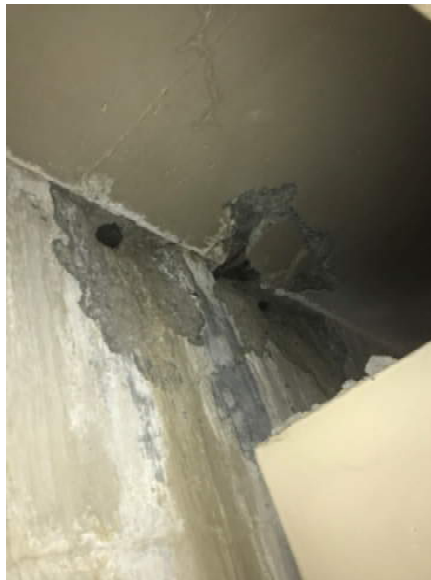
P20: Spalling concrete & delamination with stains
