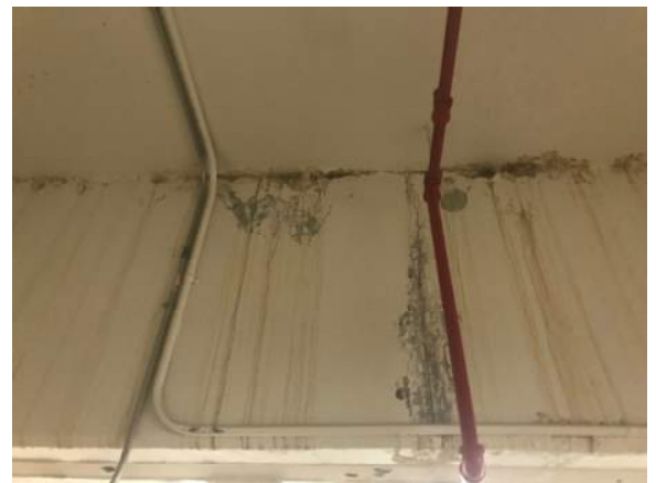
P23: Concrete cracking with stains near top of wall
