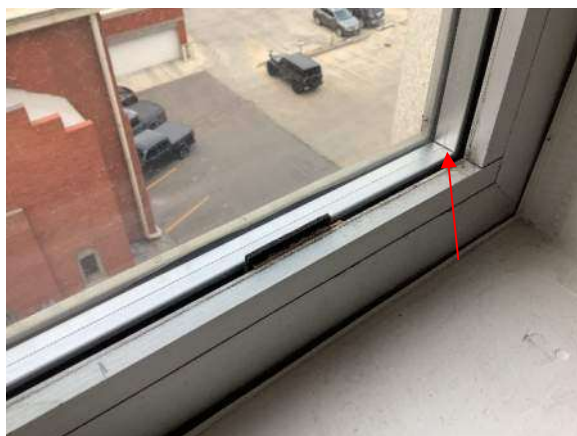
Photo #51 Recently replaced IG units typically have no spacer stamp and the spacers have cut corners (red arrow).
