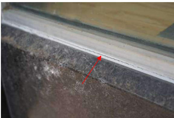
Photo #59 Cohesive failure at first floor window perimeter sealant indicated by red arrow.
