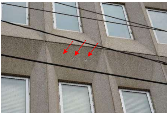
Photo #11 Minor spalling of the precast wall panels indicated with red arrows.
