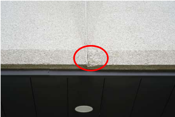
Photo #13 Small area of apparent freeze-thaw damage at the second-floor eyebrow indicated by the red oval.
