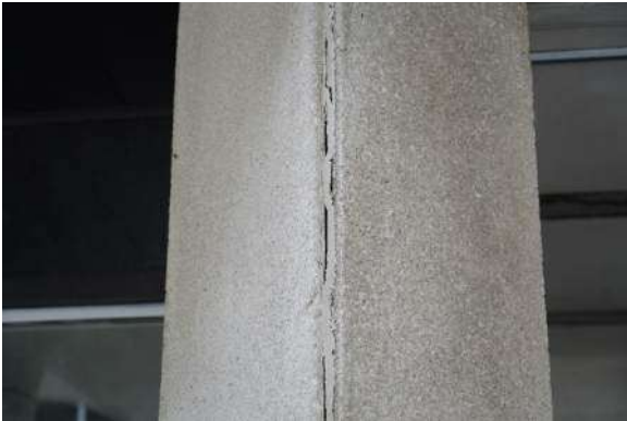
Photo #19 Separations within the joint sealant suggest that the column cover has moved.
