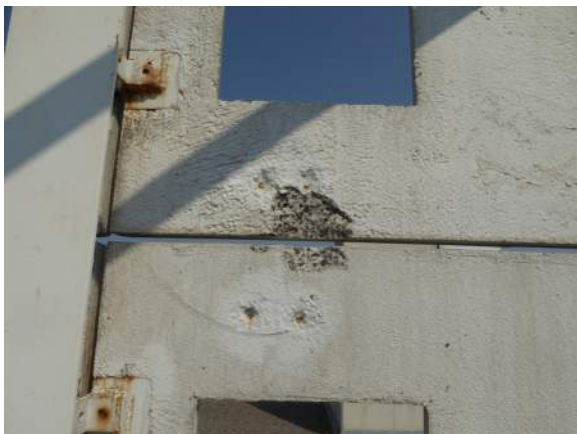
P43: Precast concrete panel joint with minor spalling concrete
