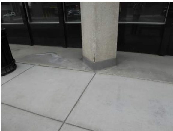
P5: weathered façade
