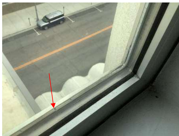
Photo #30 Original compound glazing was observed to be in very poor condition from the building interior indicated by red arrow.
