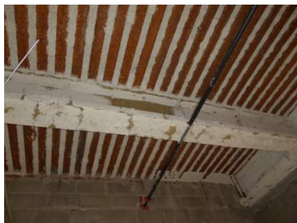
P36: Significant deck corrosion in the masonry room
