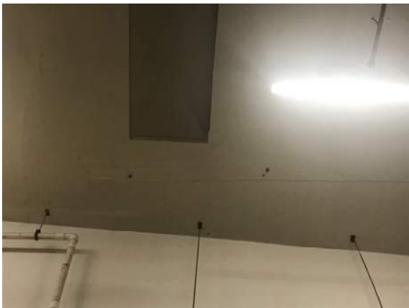
P32: concrete slab ceiling crack
