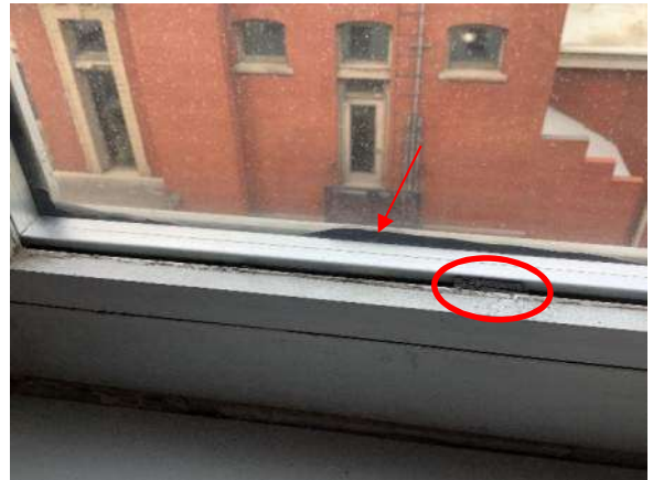
Photo #32 Butyl tape exterior glazing at recent IG unit replacement indicated by red arrow. Shim location indicated by red oval.
