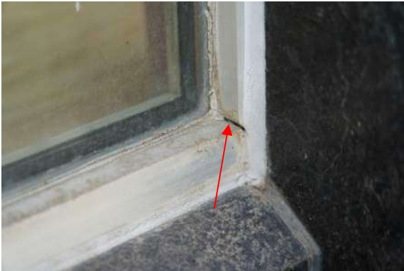
Photo #43 Open metal-to-metal joint at first floor window frame corner indicated by red arrow.
