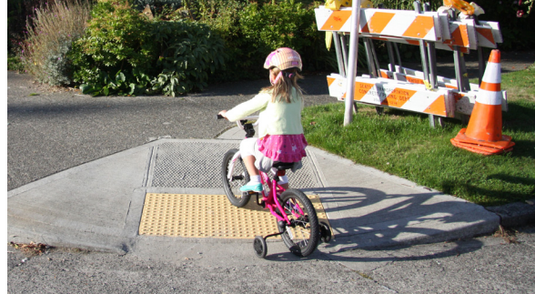
A sidewalk retrofitted with a curb ramp and a tactile warning strip
