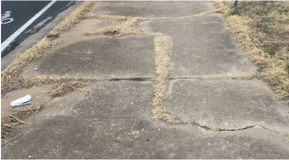
Severe cracking creates uneven and hazardous walking surfaces
