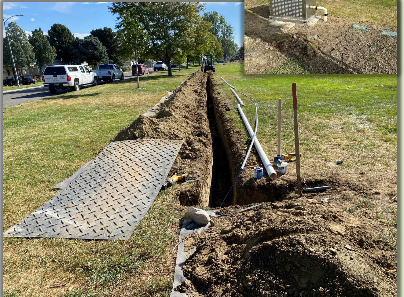
Ponderosa Park Irrigation
