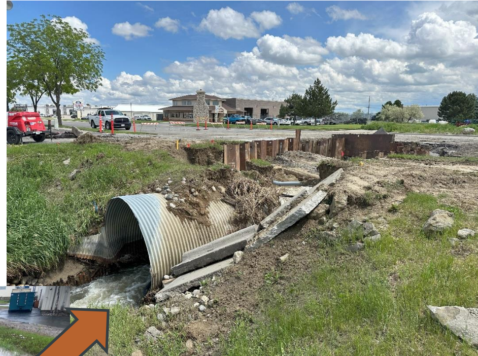
Road Failure / Emergency Replacement Project
