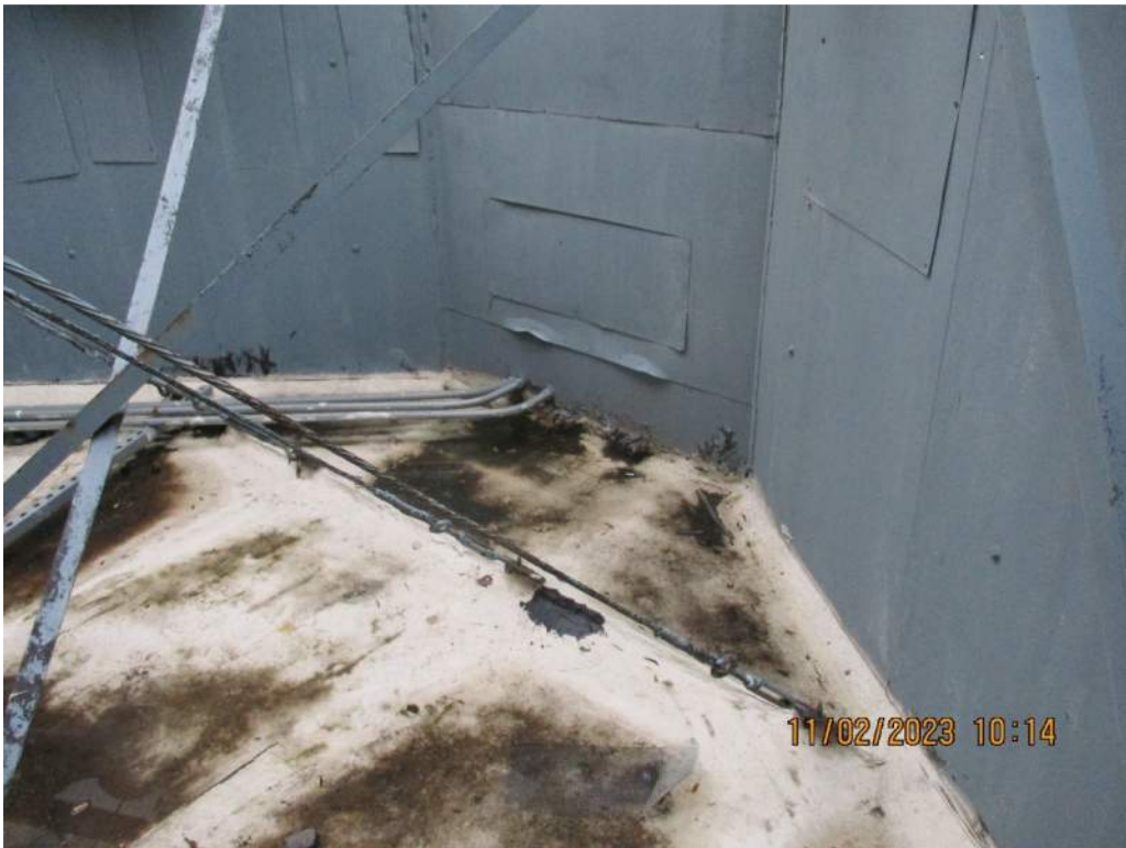
Figure 9: Deteriorated Built-Up Roofing system with Elastomeric Coating over Marquee Steel Roof Decking
