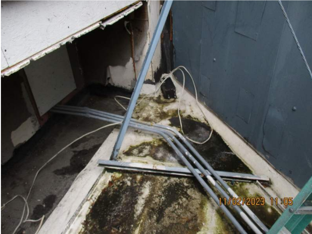
Figure 10: Deteriorated Built-Up Roofing system with Elastomeric Coating over Marquee Steel Roof Decking
