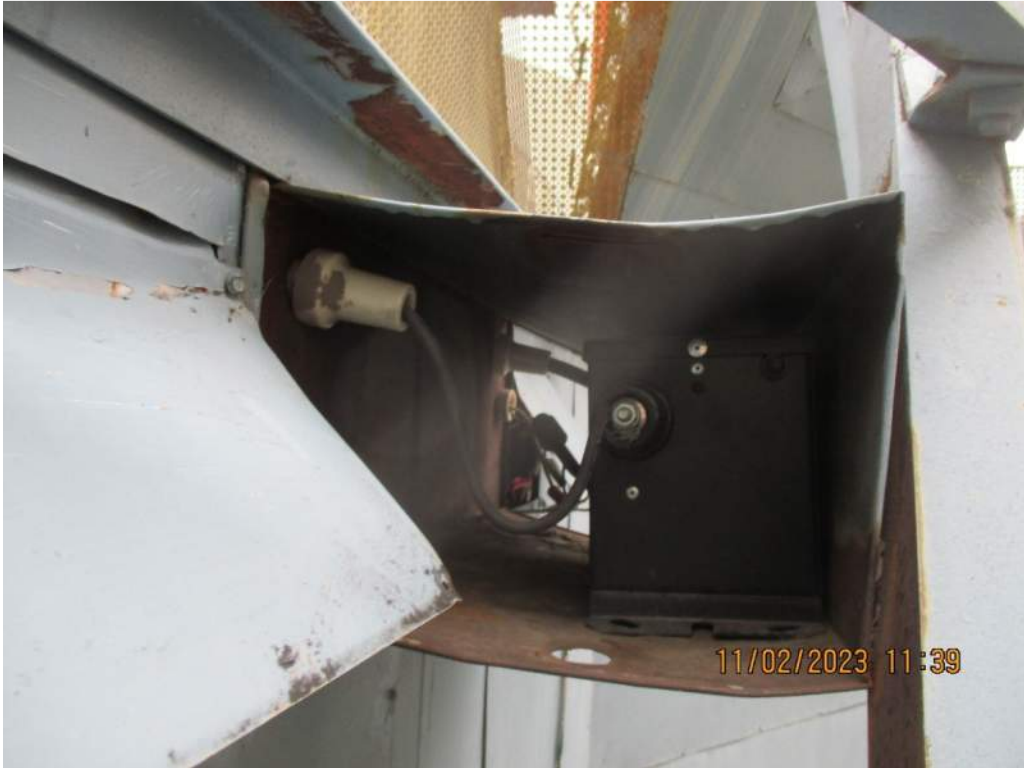
Figure 20: Typical Light Ballast Under Protective Cover at Interior Paneling
