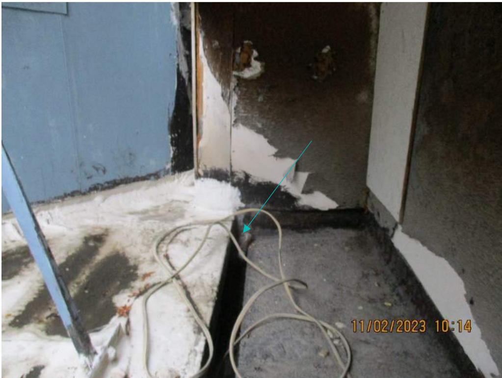
Figure 13: Location of Small Drain Outlet in East Corner of Internal Gutter
