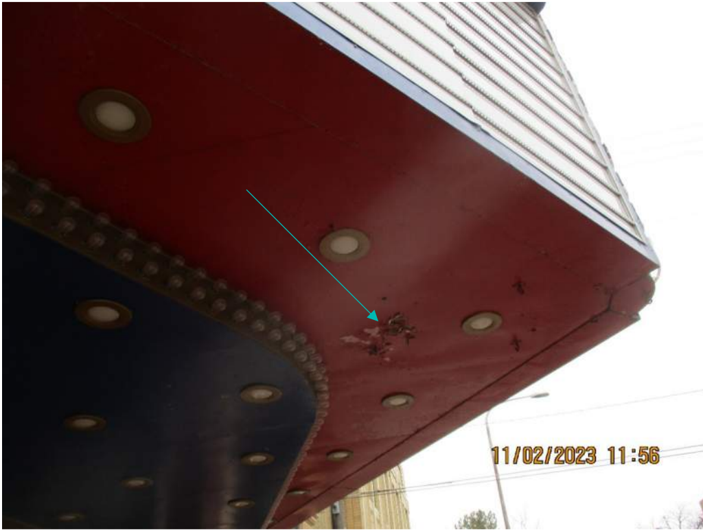
Figure 22: Deteriorated Soffit Metal Below Observed Water Leaking
