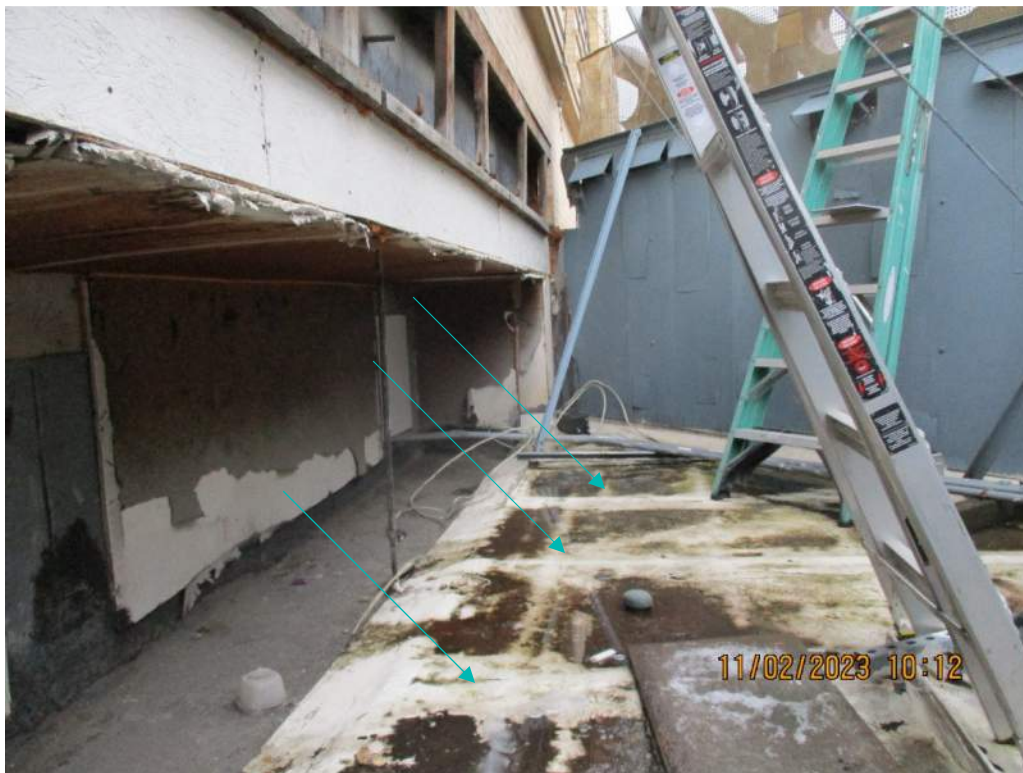
Figure 15: Locations of Underlying Structural Elements Supporting Metal Roof Decking and Exterior Marquee Paneling (Approximately 4' O.C.)
