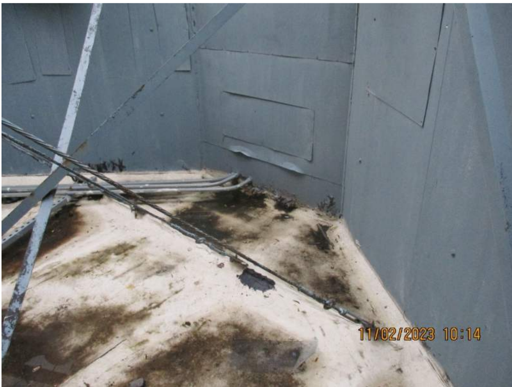
Figure 9: Deteriorated Built-Up Roofing system with Elastomeric Coating over Marquee Steel Roof Decking
