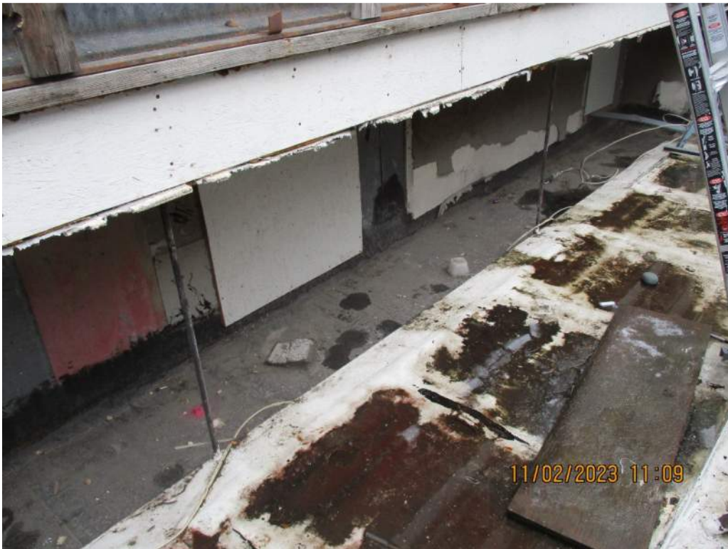
Figure 11: Deteriorated Built-Up Roofing at South End of Marquee Along Transition to Internal Gutter
