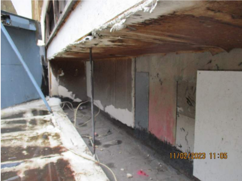
Figure 14: Condition of Deteriorated Wall Substrate Boards Above Internal Gutter
