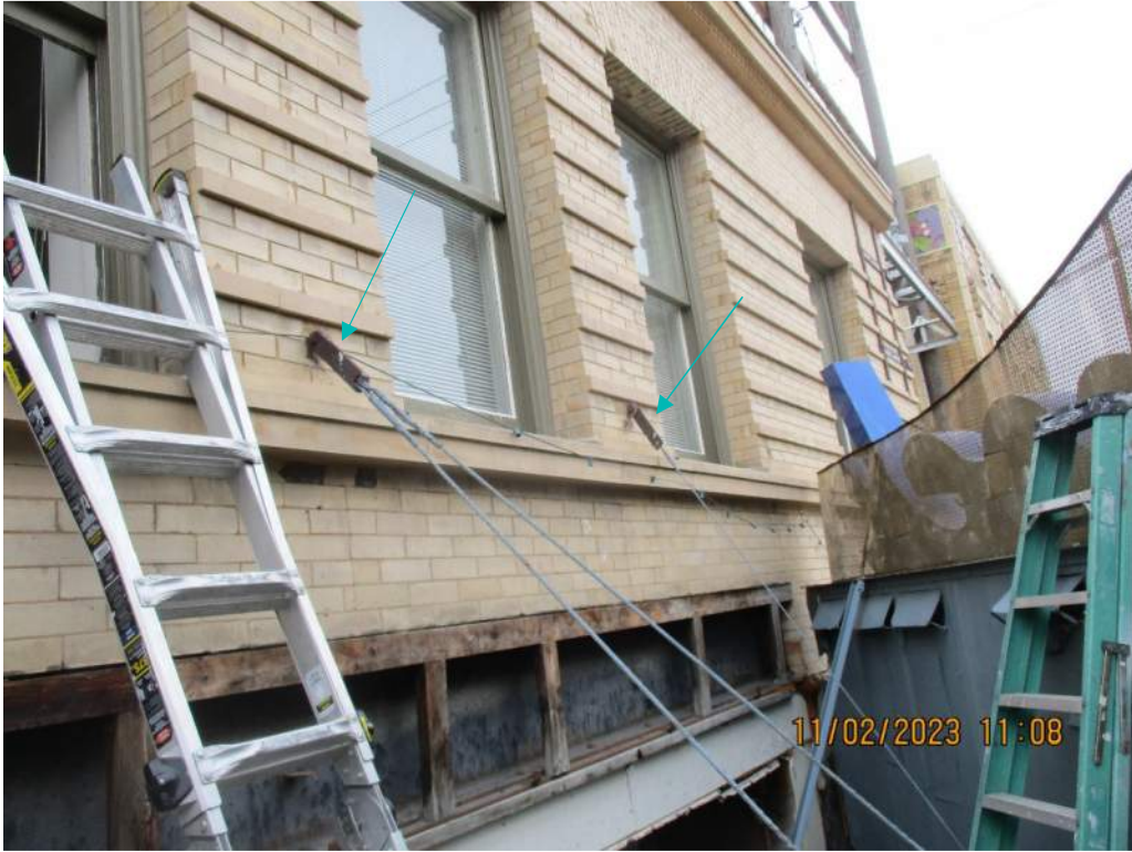
Figure 18: Cable Tie Back Connections at Exterior Wall
