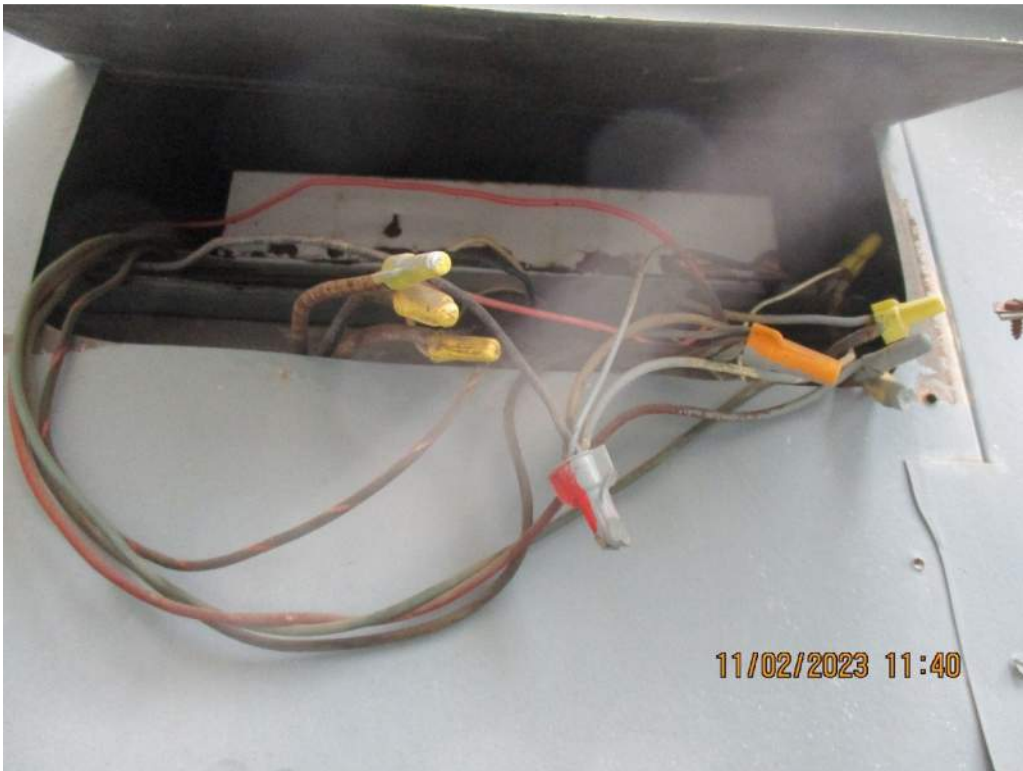
Figure 19: Electrical Wiring Within Interior Paneling Access Locations - Typical
