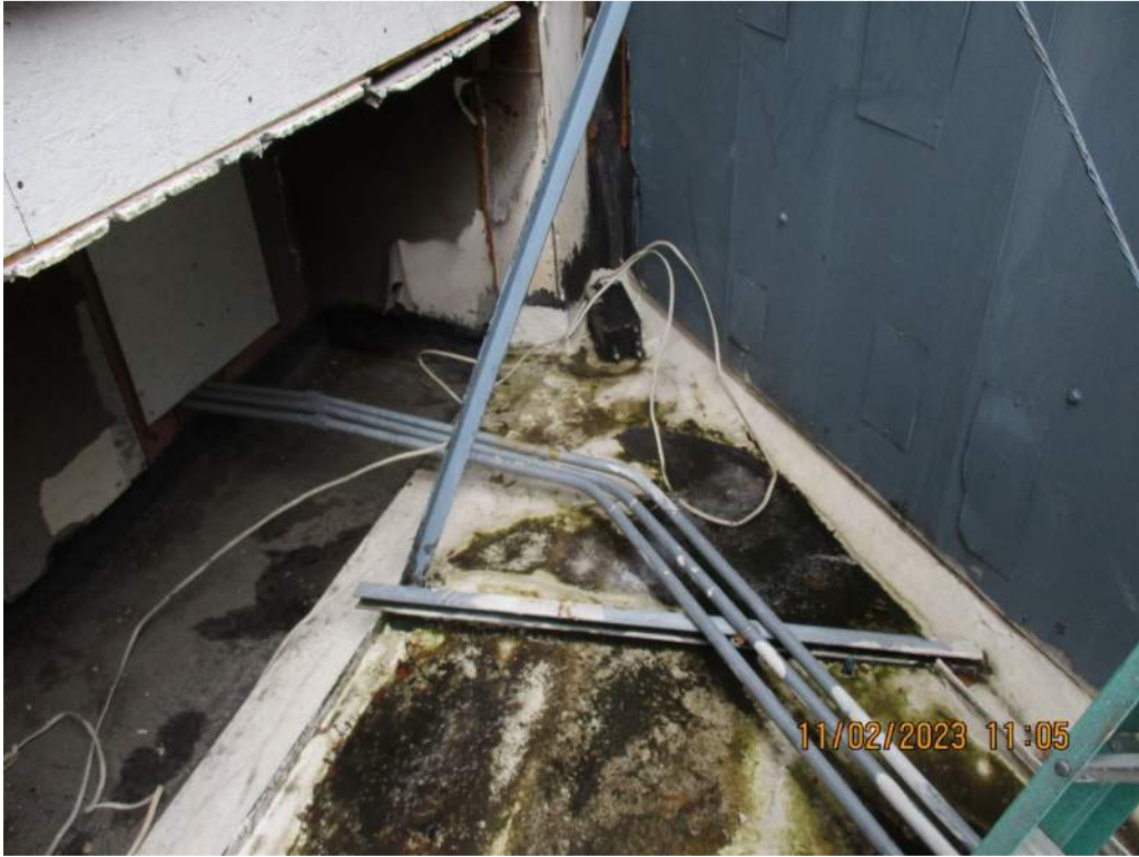
Figure 10: Deteriorated Built-Up Roofing system with Elastomeric Coating over Marquee Steel Roof Decking
