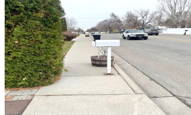
Vegetation should be trimmed to maintain minimum clear width
