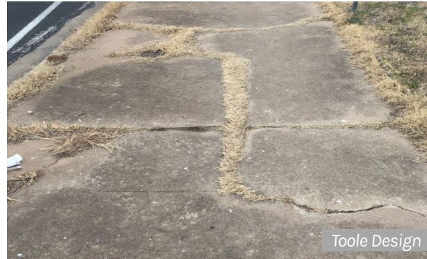
Severe cracking creates uneven and hazardous walking surfaces
