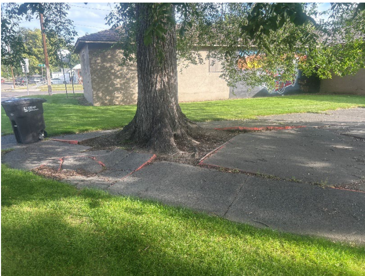
Damaged, unsafe sidewalks in South Park.
