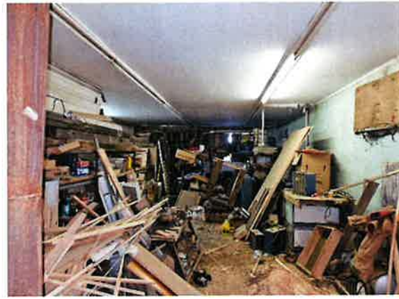
12) Photograph taken inside the east end of the building, looking east. Sheetrock ceiling contains <1% asbestos.
