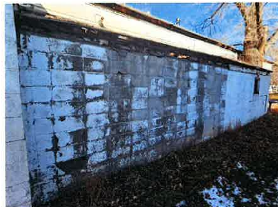
4) Meat House and Lockers building looking northeast. White peeling paint on CMU tested negative for lead.
