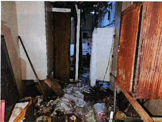
14) Photograph showing the poor conditions within the building that may include biological hazards.
