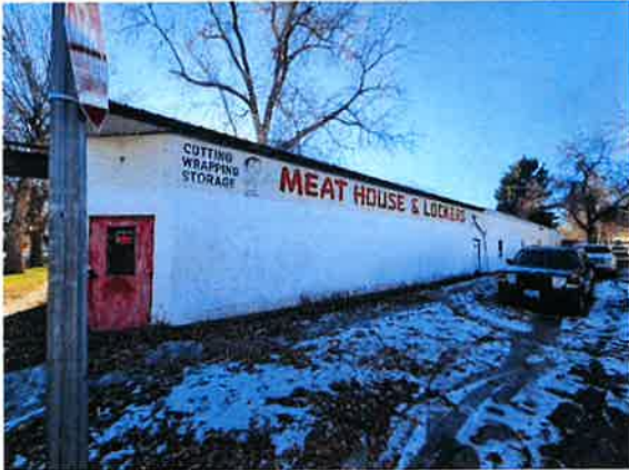
1) Meat House and Lockers building looking southwest. Select areas of white paint on CMU tested positive for lead.
