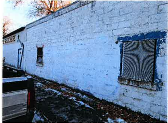
7) Close-up of the southwest exterior corner of the Meat House and Lockers building looking east. White paint on CMU, and blue and red paint on wood tested negative for lead.
