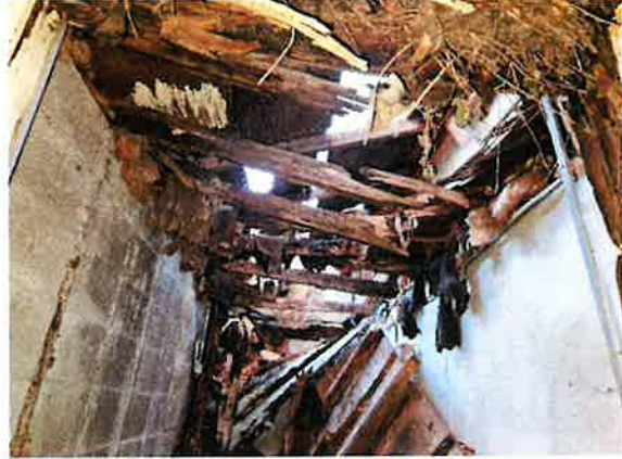
11) Close-up of collapsed roof looking west from the south storage area.
