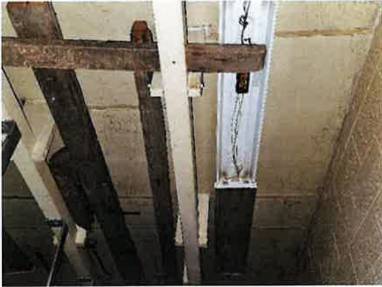
17) Photo of one type of light ballast presumed positive for PCB's.
