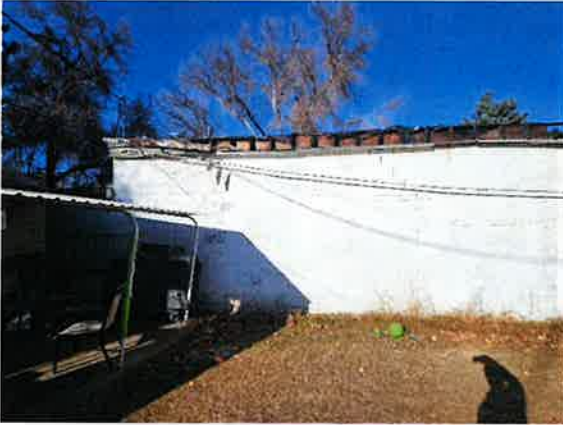
5) Meat House and Lockers building looking north at the west end of the building. White paint on CMU tested negative for lead.
