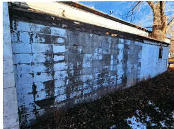
4) Meat House and Lockers building looking northeast. White peeling paint on CMU tested negative for lead.
