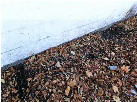
18) North side of the building underneath the areas that tested positive for lead. Confirmed the LBP is above the concrete sidewalk.
