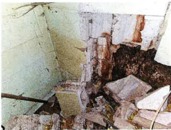
10) Close-up of damaged CMU wall looking west from the south storage area.
