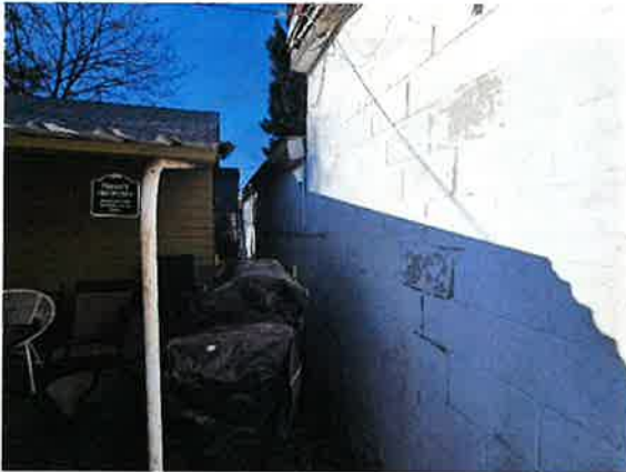
6) Close-up of the southwest exterior corner of the Meat House and Lockers building looking west. White paint on CMU tested negative for lead.
