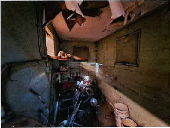
9) Water damaged sheetrock ceiling confirmed in the south storage area. Green paint on CMU tested negative for lead.
