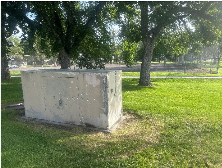
Damaged electrical infrastructure in South Park.
