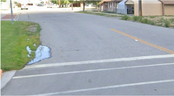
Improper drainage and missing curb, gutter or sidewalk on Fifth Avenue South near 27 th Street, right at the entrance to Downtown Billings.
