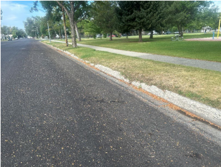
Deteriorated curb and gutter at Highland Park.
