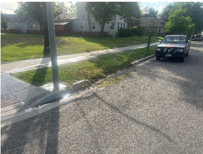
Deteriorated curb and gutter near the intersection of 4 th Avenue South and South 31 st Street.
