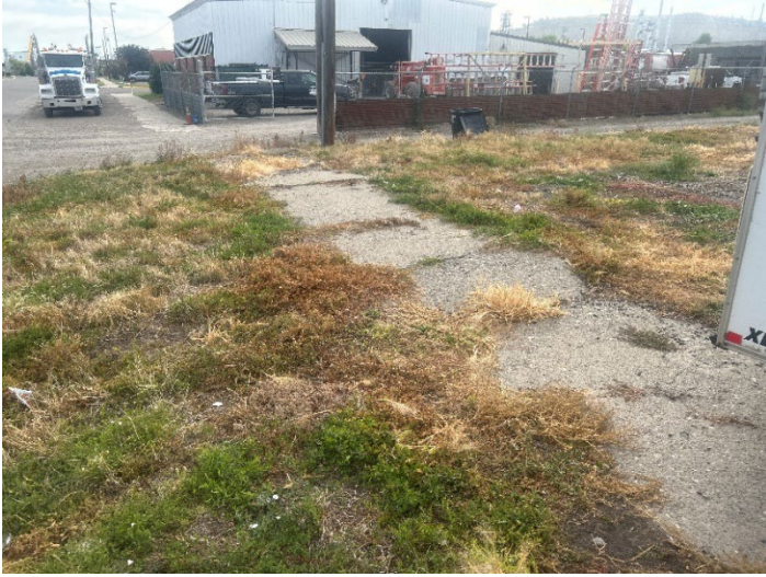
Deteriorated sidewalk near the intersection of 3 rd Avenue South and South 25 th Street.
