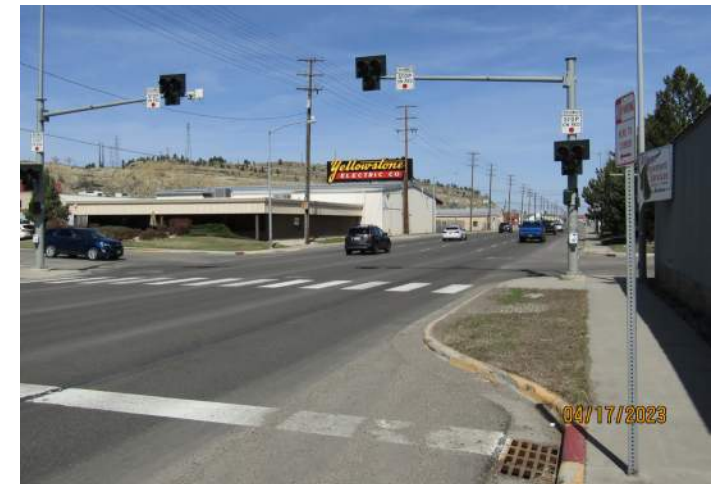
Pedestrian Hybrid Beacon (PHB). Source: DOWL
