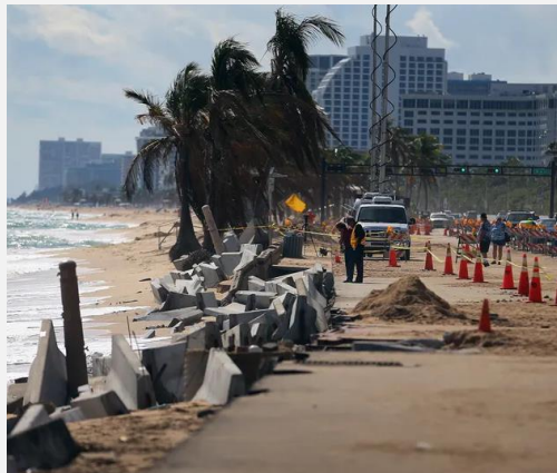
Fort Lauderdale – A1A Washout
