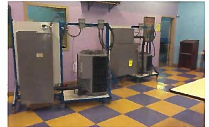
HVAC equipment in a general meeting room
