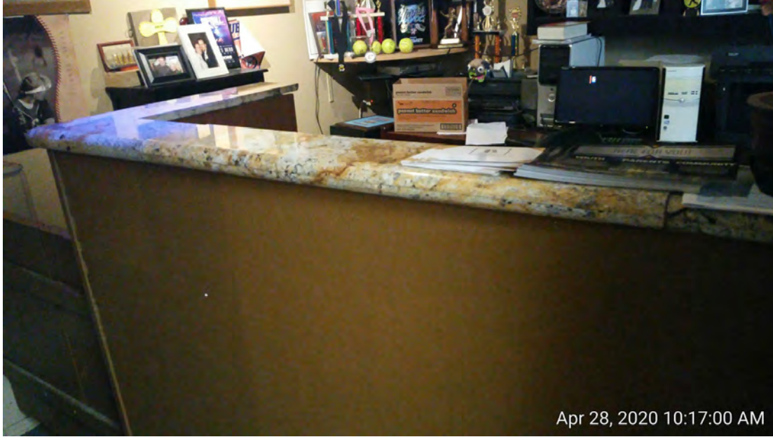
Service counter is not accessible. C
