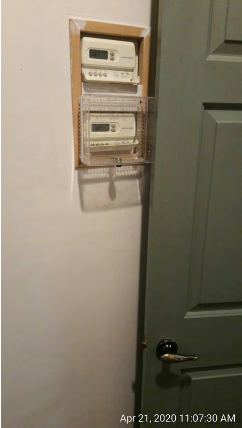
Thermostat controls exceed allowable reach ranges. T
