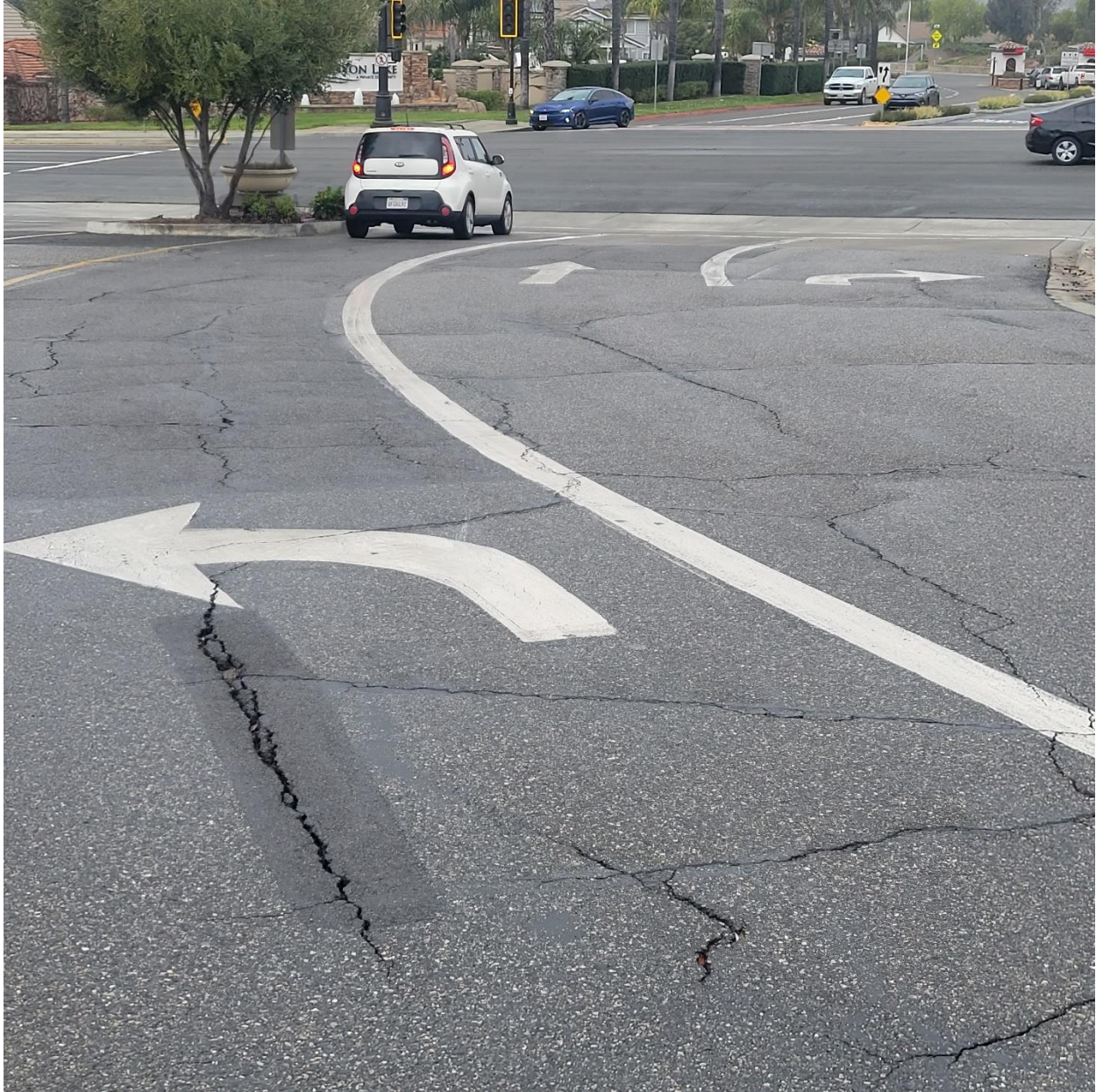
Exhibit 1 - View of the lane markings on the South approach leg (Northbound) of the Canyon Lake Drive South/Towne Center at Railroad Canyon Road intersection.
