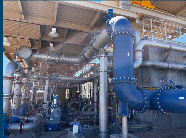
Chandler Reclaimed Water Interconnect Facility – Opened October 2024
