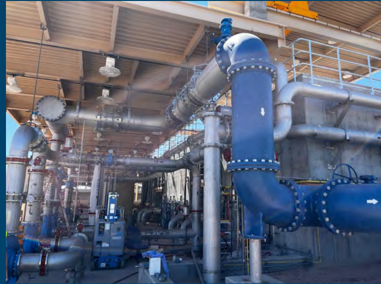
Chandler Reclaimed Water Interconnect Facility – Opened October 2024
