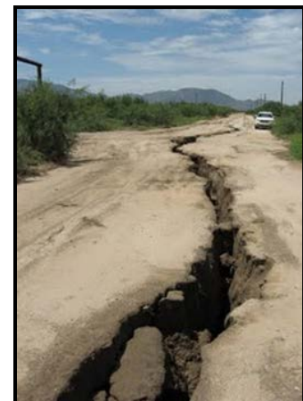
Recently developed earth fissure near Willcox. (Arizona Geology, 2011)
