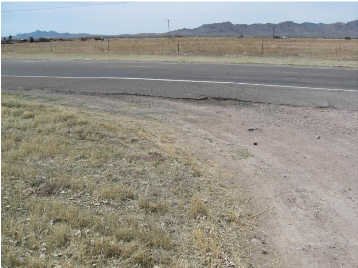
The access onto Fort Grant, showing the existing wear.
