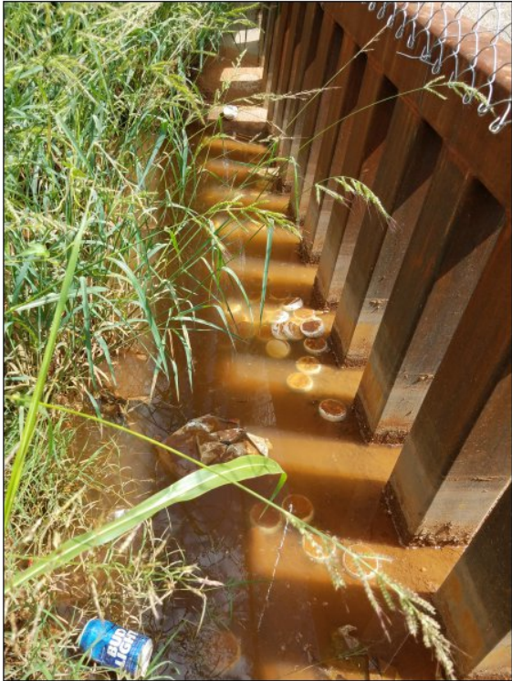
Photo 1 – Sewage at POE
