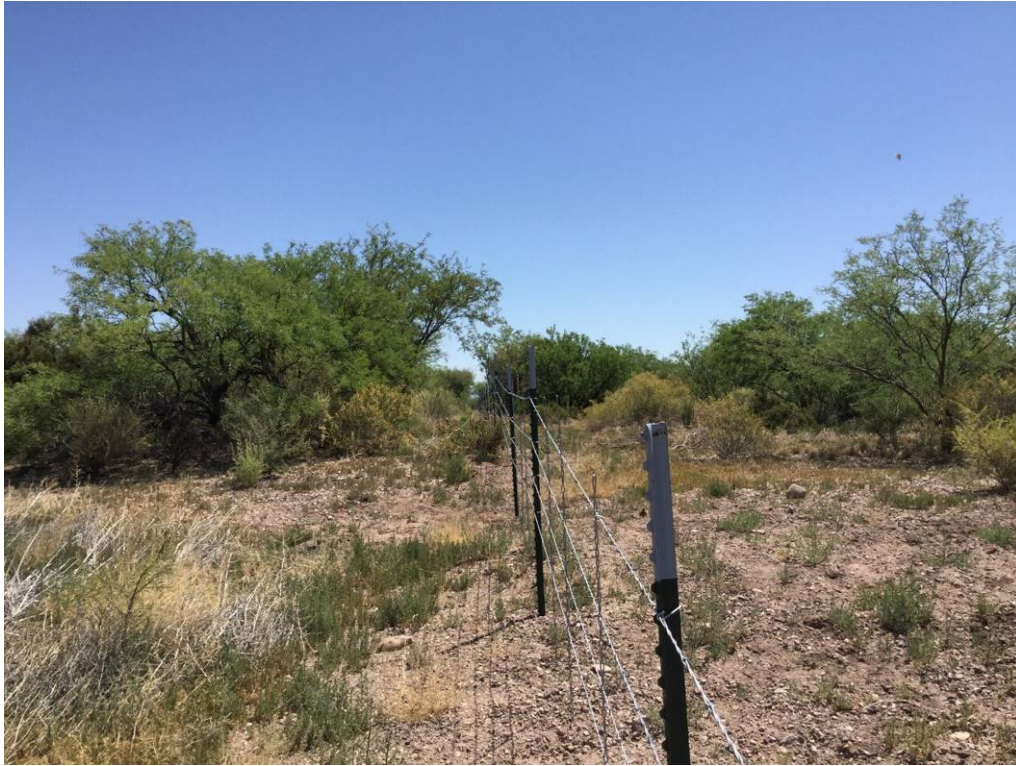
PHOTO 9: LOOKING EAST ALONG THE INTERIOR FENCE ALONG NORTH BANK CUT. (PHOTO POINT 3)
