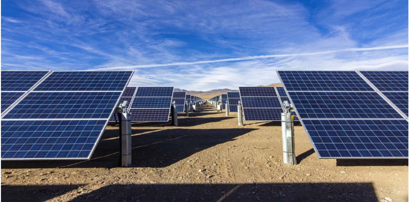
Figure 7: Typical ground mounted solar field
