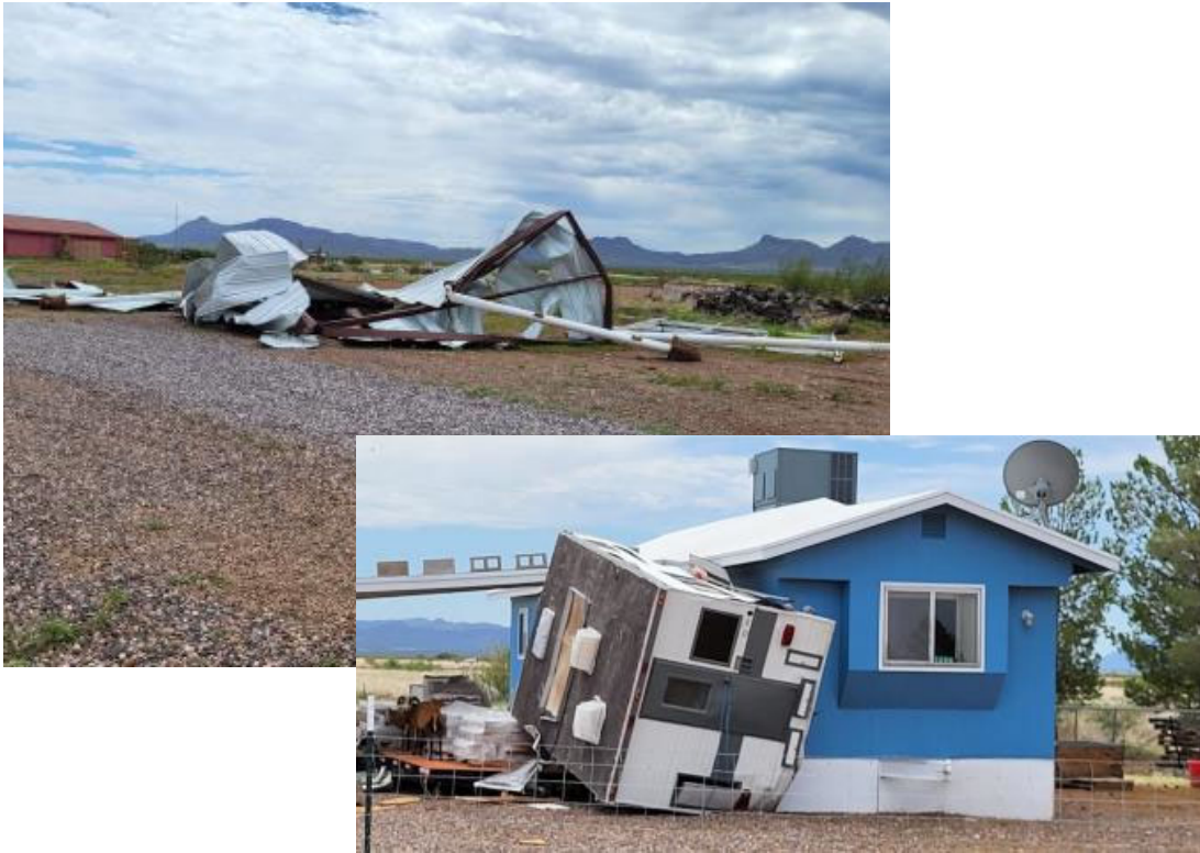
Figure 5.3-32. Damage from Wind Event July 19, 2022
