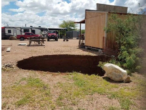
Figure 5.3-1. Sinkhole Mine Collapse in Tombstone
