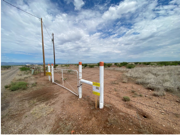
Gated entry to the gas line easement
