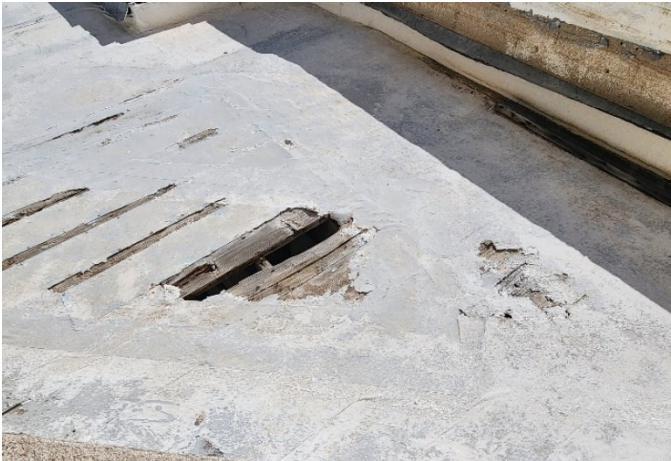
Rotted Roof Decking Around Dome
