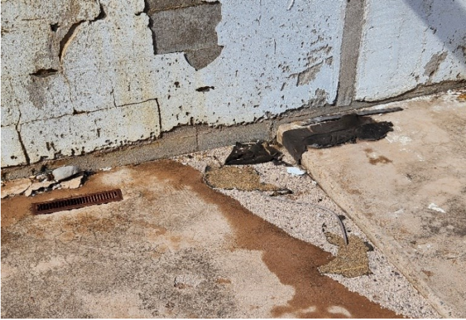
Concrete Slab Portion Depressed Down
