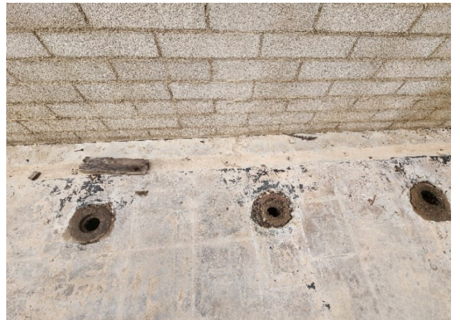
Main Restroom Cast Iron Plumbing
