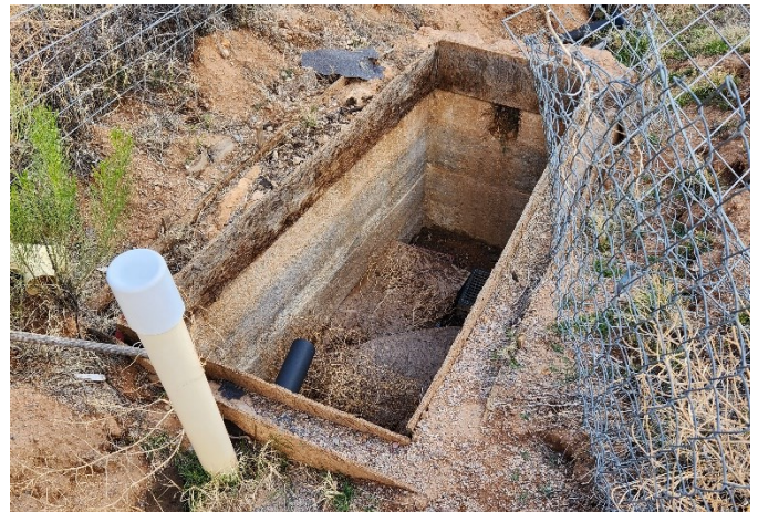
Onsite Septic System
