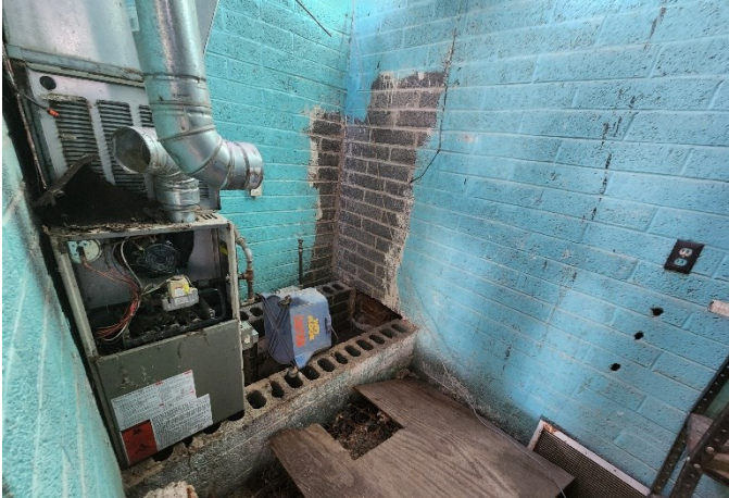
Girls Dormitory Furnace
