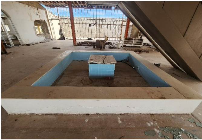
Main Lobby Fountain
