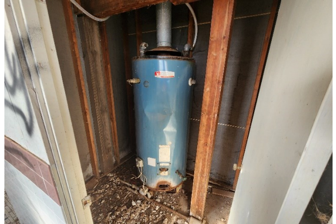
Girls Dormitory Water Heater
