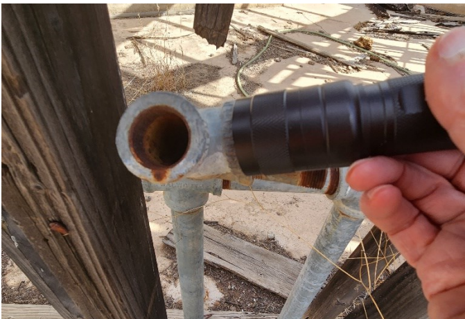
Galvanized Supply Piping
