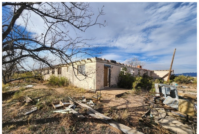
Boys Dormitory Exterior Debris
