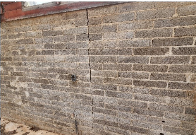
Masonry Structural Vertical Crack
