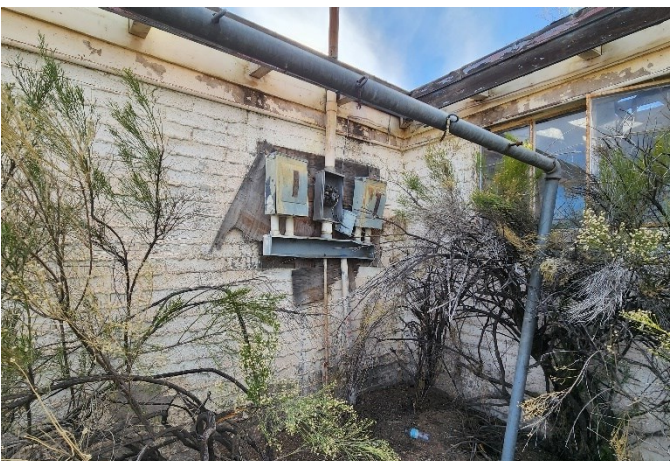
Boys Dormitory Exterior Electrical Panels
