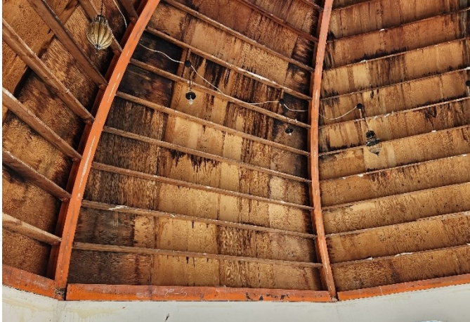
Interior Dome Water Stains
