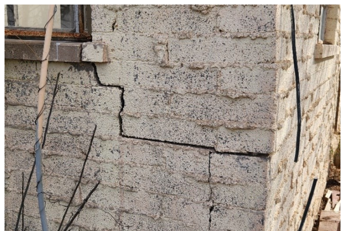
Boys Dormitory Crack in Exterior Wall
