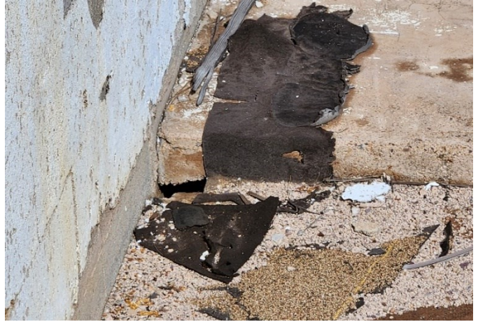
Concrete Slab Portion Depressed Down
