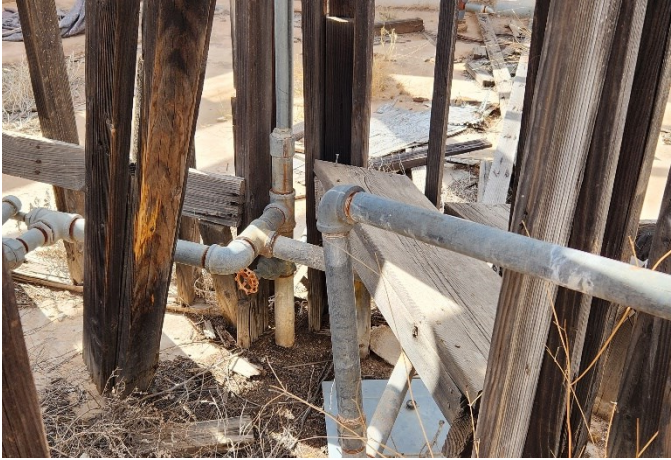
Galvanized Supply Piping
