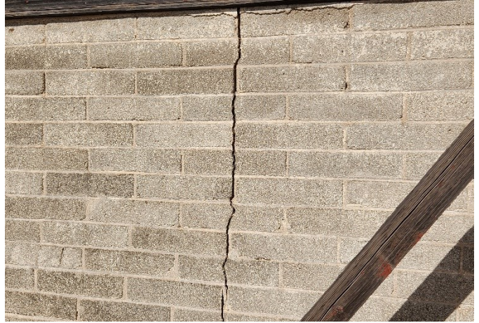
Structural Vertical Crack
