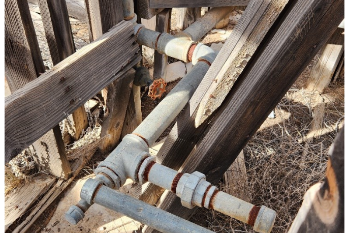
Galvanized Supply Piping
