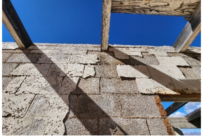
Deteriorated Masonry Finish
