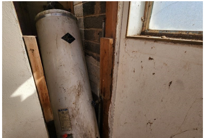
Boys Dormitory Water Heater
