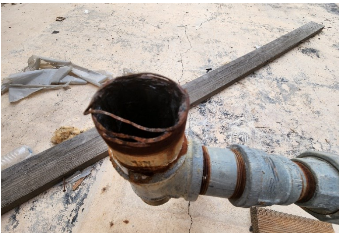
Exposed Galvanized Pipe in Restroom
