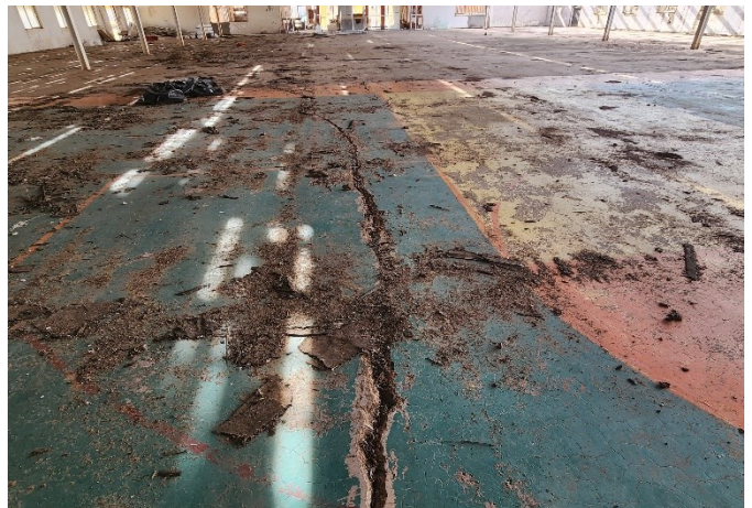
Severely Cracked Slab in Auditorium
