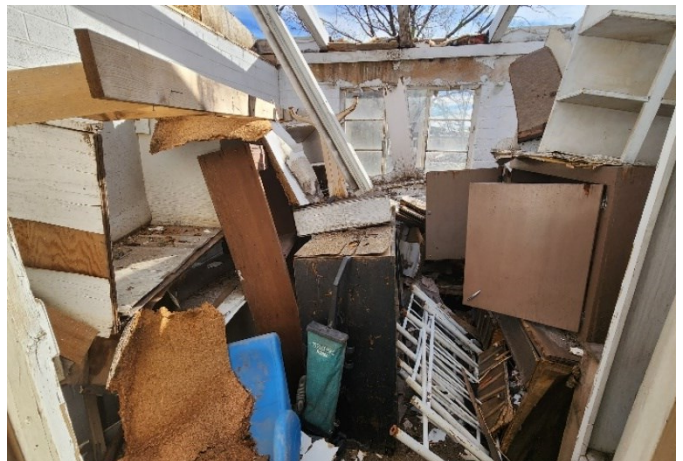
Boys Dormitory Room Full of Debris
