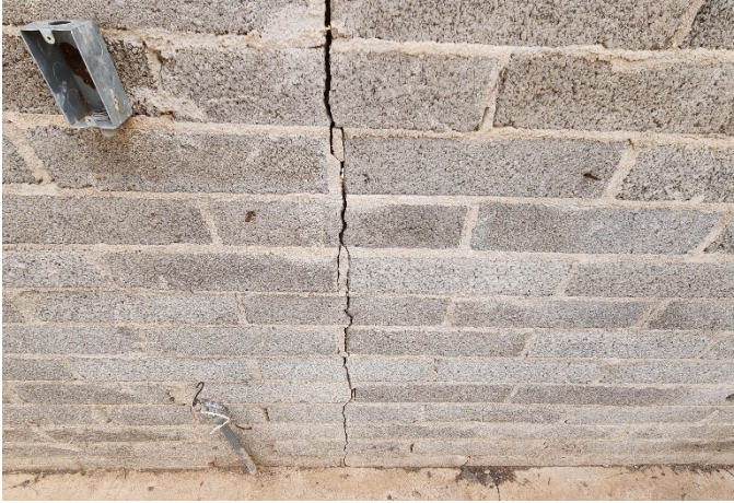
Masonry Structural Vertical Crack
