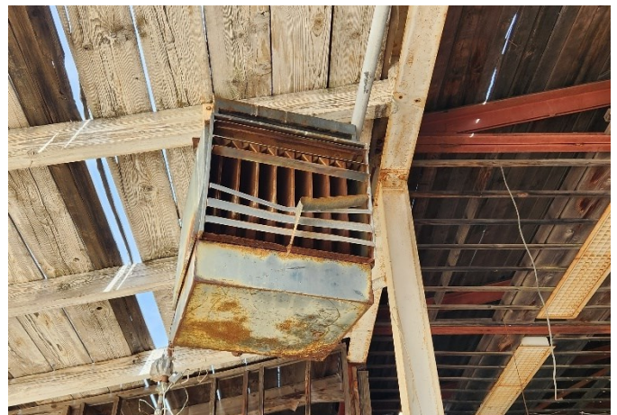
Ceiling Mounted Gas Furnace
