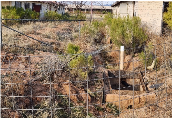
Onsite Septic System
