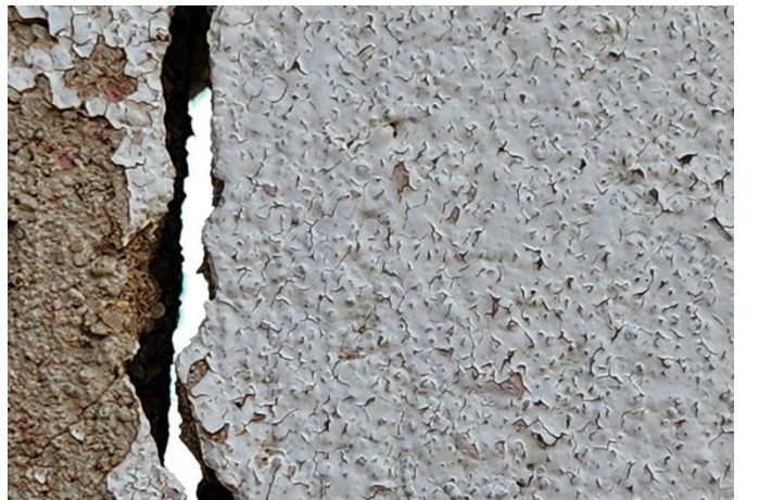
Closeup View of Masonry Vertical Crack
