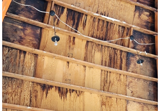
Interior Dome Water Stains
