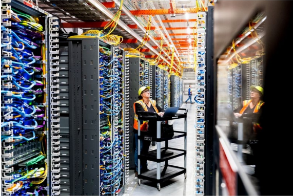
A technician works in a data center. | Noah Berger/Getty Images via Amazon Web Services
