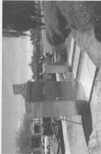
Cabinet and meter pedestal at 91st Ave and Union Hills
