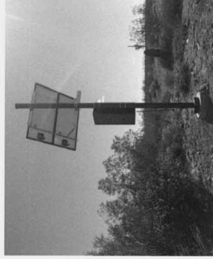
Solar panel for monument sign at Vistancia
