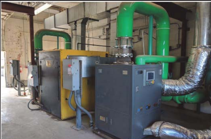
Current WRF Blower System
