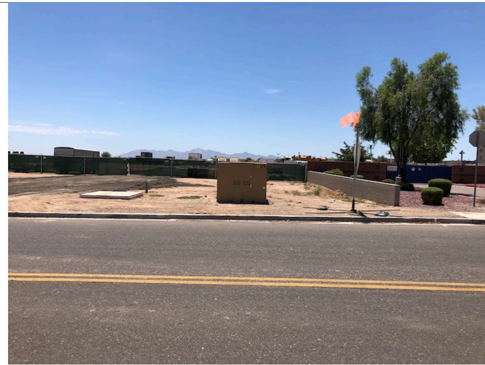
PHOTO 2: EXISTING ELECTRICAL TRANSFORMERS
