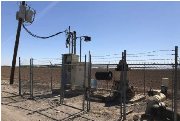
View of the irrigation supply well and pump located along the northern site boundary just east of the NWC of the subject property.
