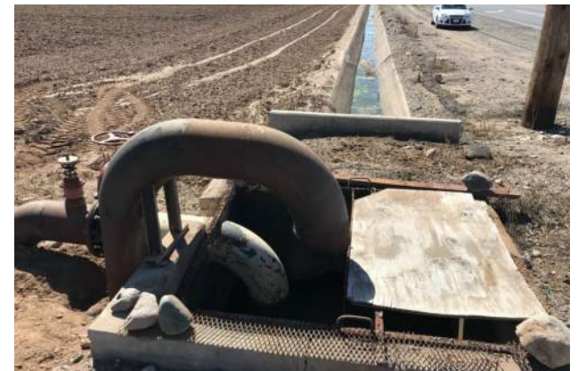
View of the irrigation piping near the NWC of the subject property.
