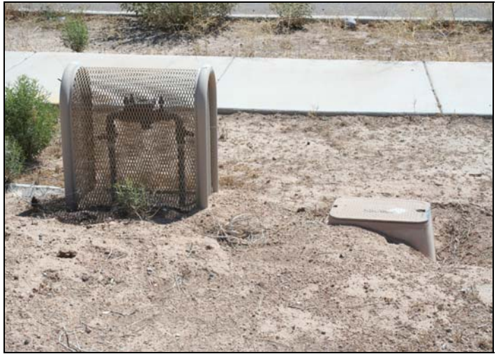
This is a view of water service available to the site.
