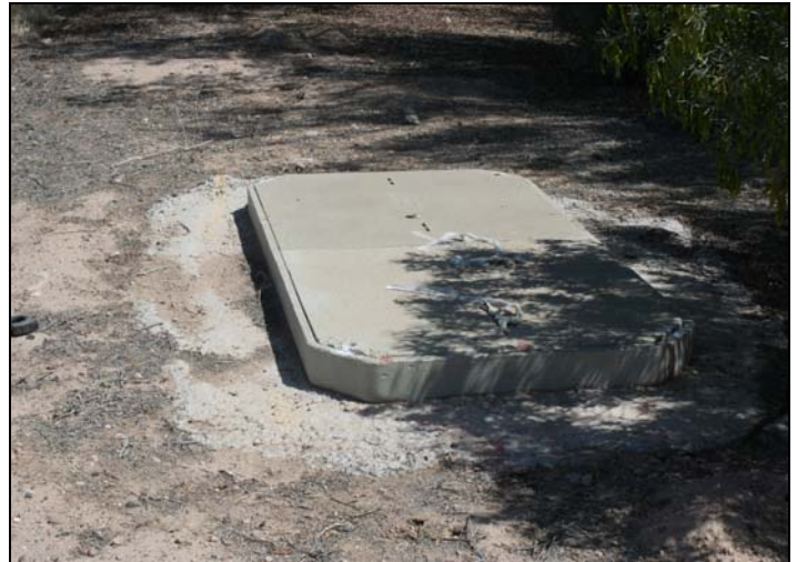
This view is of a newly installed underground utilities service vault on the site.
