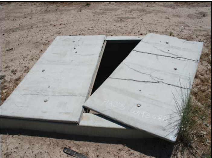
This is a view of an underground utility service vault.
