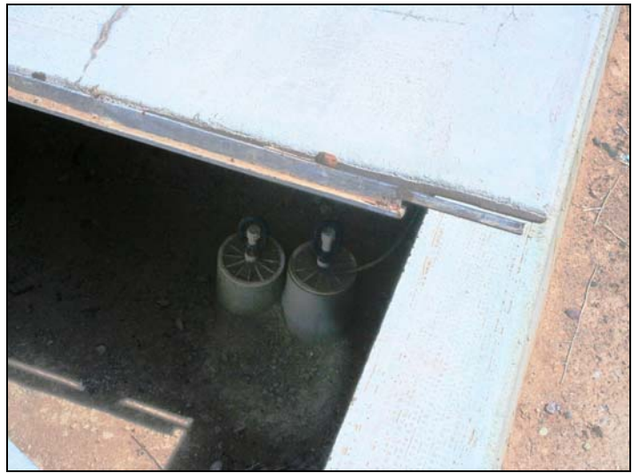
This is a view of the interior of the underground utility service vault.
