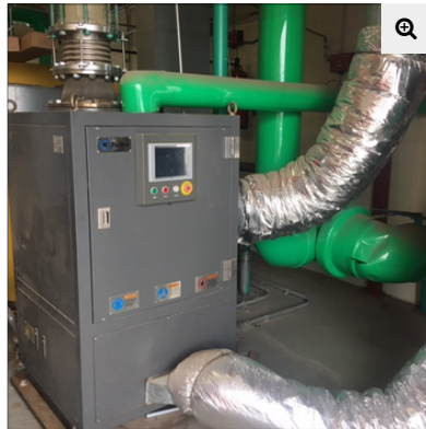
Wastewater Process Equipment
