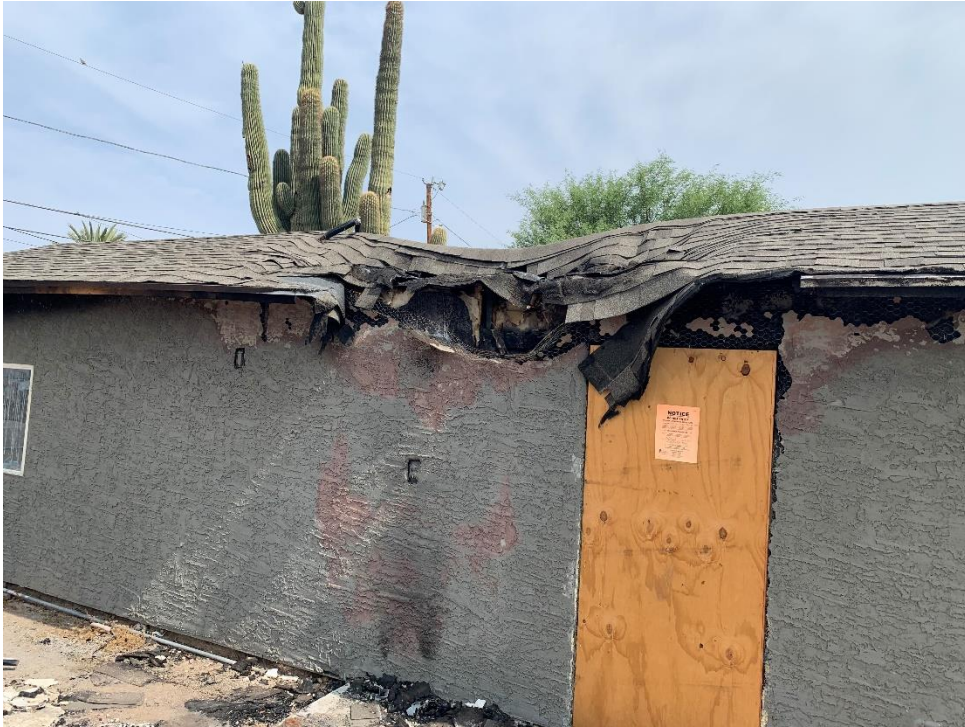
Dwelling unit Number 1, partial roof collapse.
