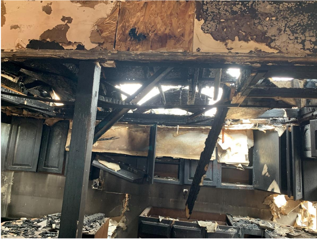
Structural damage to main structure, partial roof collapse.
