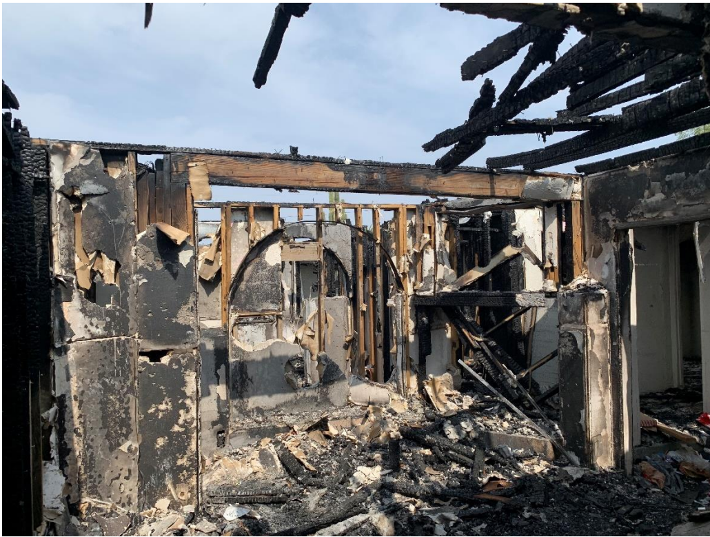
Rear view of main structure. Complete roof collapse and wall collapse.
