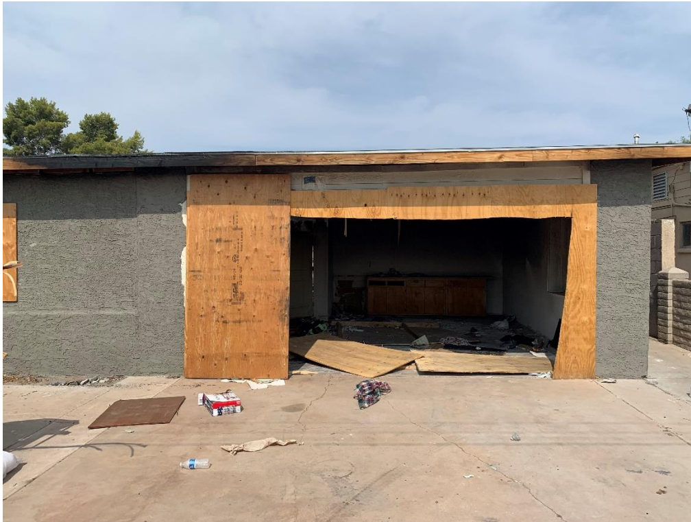
Front View of main structure. The garage area is no longer secured.
