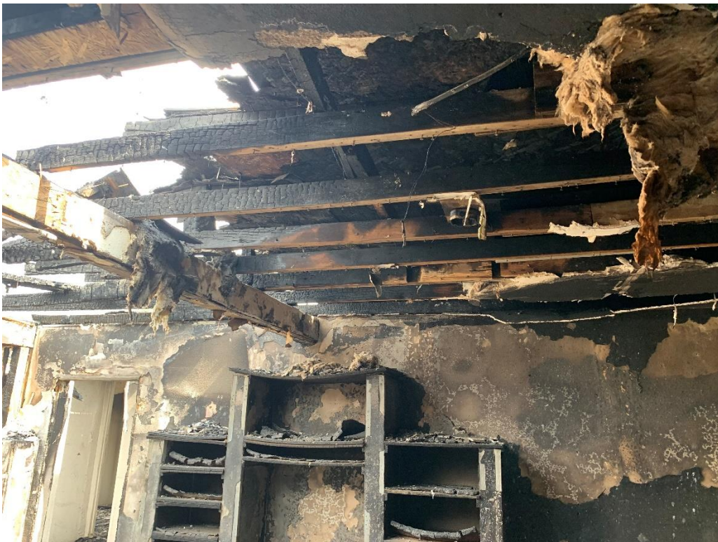
Structural damage in main structure
