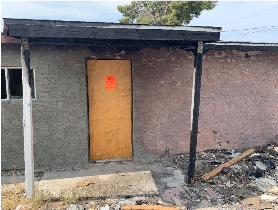
Dwelling unit number 2 on the southwest side of property. This unit has fire damage and is unsecured.
