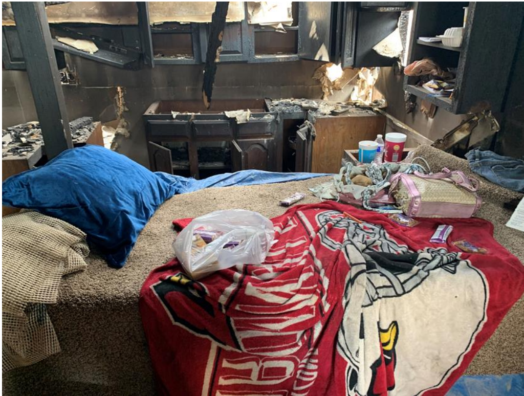
Kitchen of main structure. Evidence of unknown individuals living in structure.
