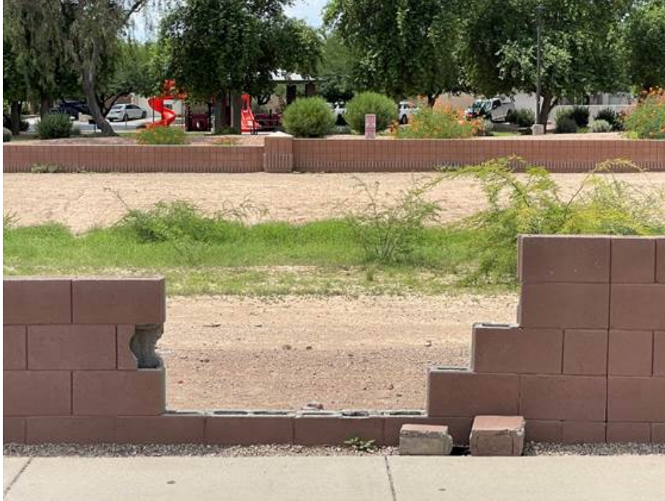
Looking west on 126th Ave more damage to same pony wall just replacing what was already there (not a part of this application just as reference to damage sustained).
