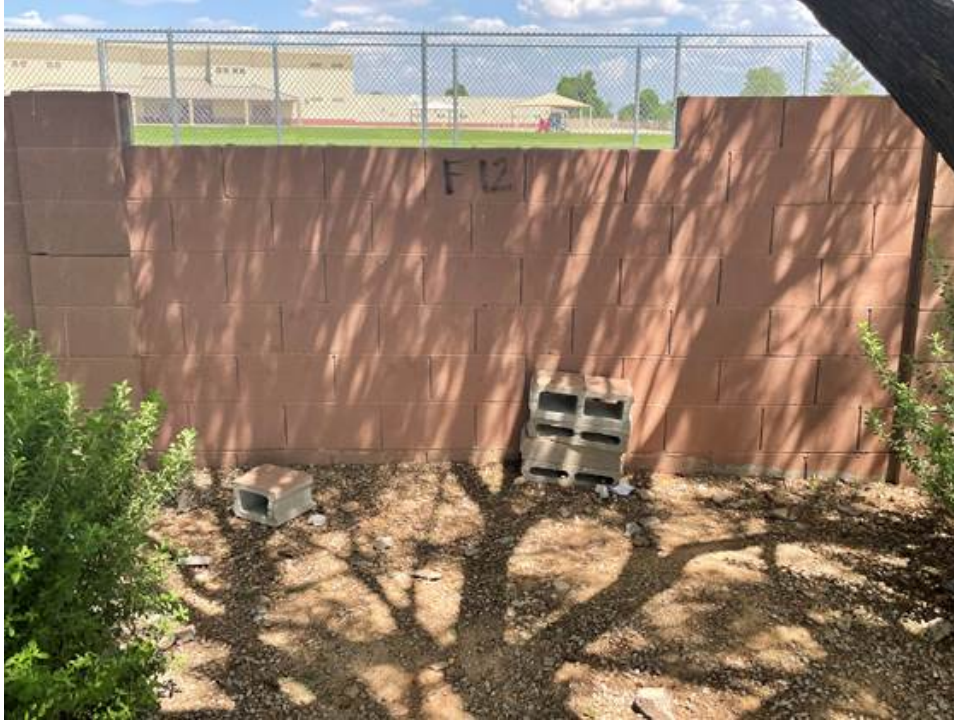
Close up of damage to a recently repaired section.
