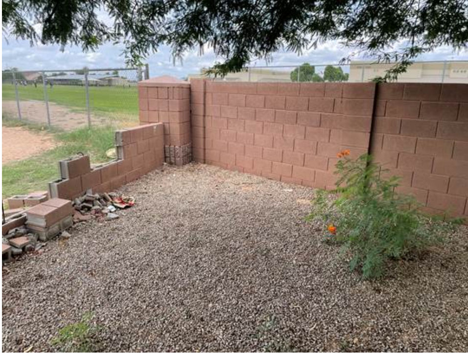
Looking west from 126th Ave showing all damage to section regarding to permit.
